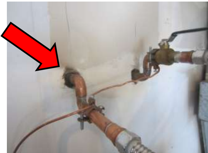
Holes in drywall
