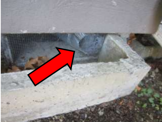
Dryer vent does not extend out from crawlspace
