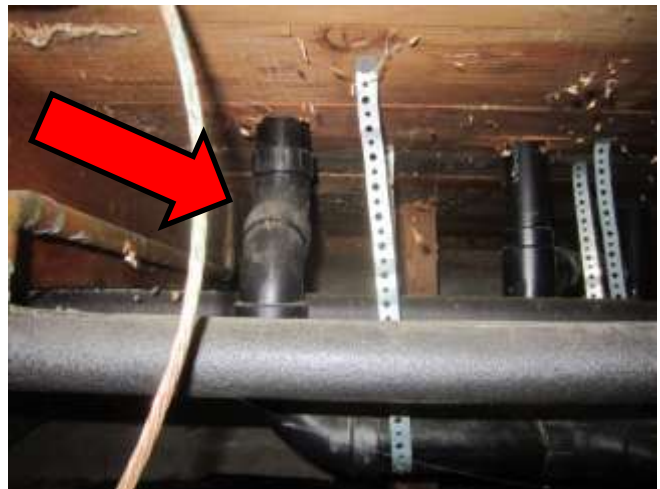
ABS waste lines beneath bathrooms
