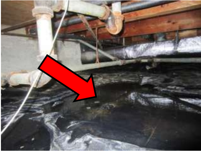
Standing water beneath Main bathroom
