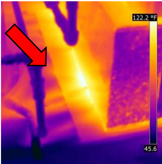
Air leakage at furnace
