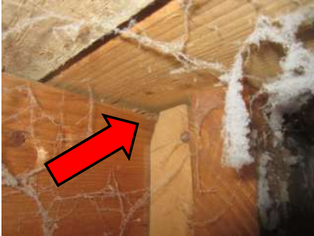
Floor beam below Master bedroom is tipped upwards at the splice creating a floor bump
