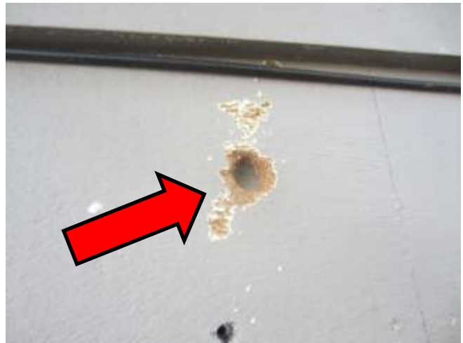
Hole in Siding
