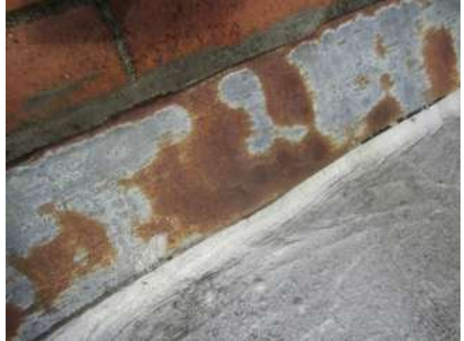
Counter flashing at chimney A coat of rust kill-proof paint would help prevent further deterioration
