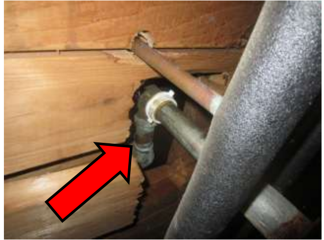
Water drips from tub drain area
