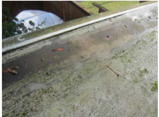
Moss build up and no coating at East roof area
