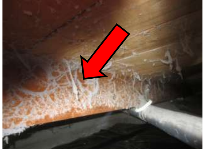
Lint inside the crawlspace
