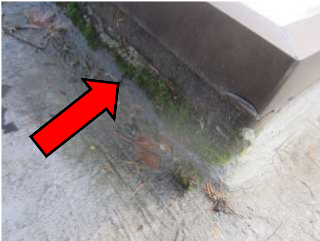
Moss build up at the upper side of the skylights
