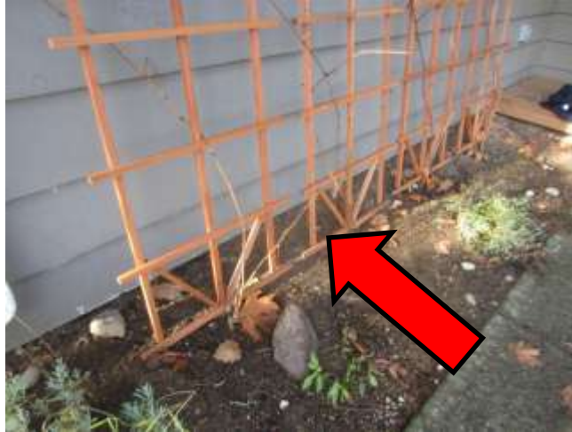
Ground in contact with siding (typical)
