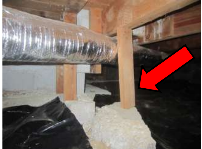
Support post is placed on concrete debris near the West side of the chimney area. Wood is not pressure treated and is at an angle
