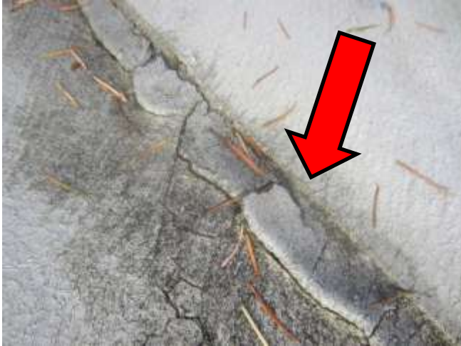
Recommend seal gaps at valley
