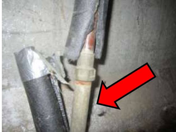
Galvanized supply pipe Unable to verify proper galvanized to copper pipe connection. Improper connection will result in corrosion of the pipe
