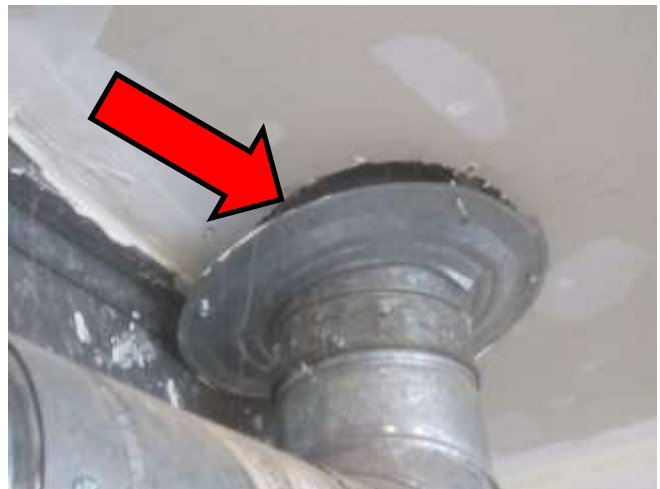
Loose flue collar
