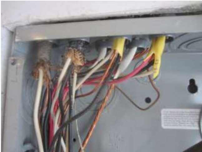
Wiring is a mix of 2 and 3 (grounded) branch wiring
