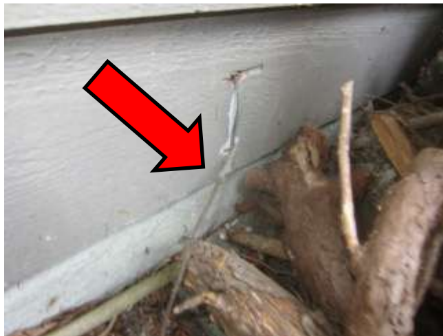
Exterior grounding wire
