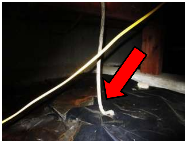
Presumed abandoned electrical wire in crawlspace Yellow wire should be secured to framing above
