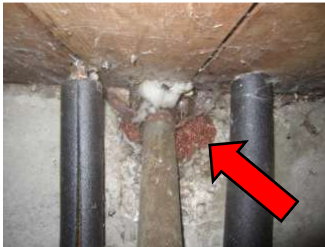
Metal mesh is placed beneath Kitchen sink to deter rodents from chewing into cabinet above
