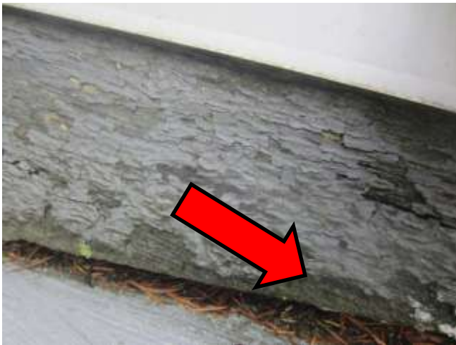
Wood rot at fascia board
