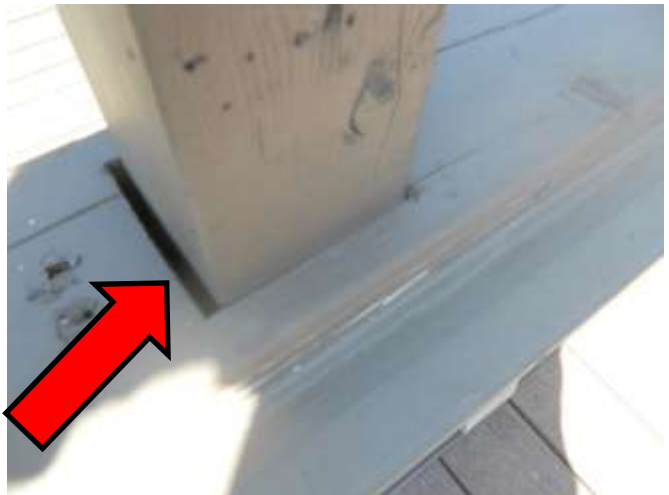
Gaps at posts at deck rail could lead to wood rot
