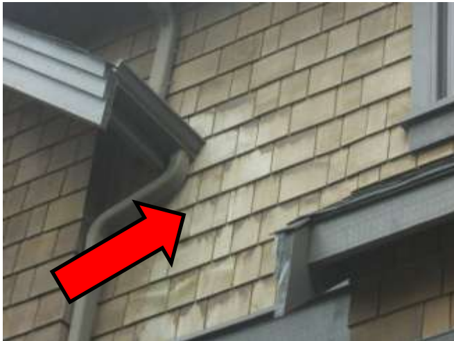
Siding stain shows evidence of spillage
