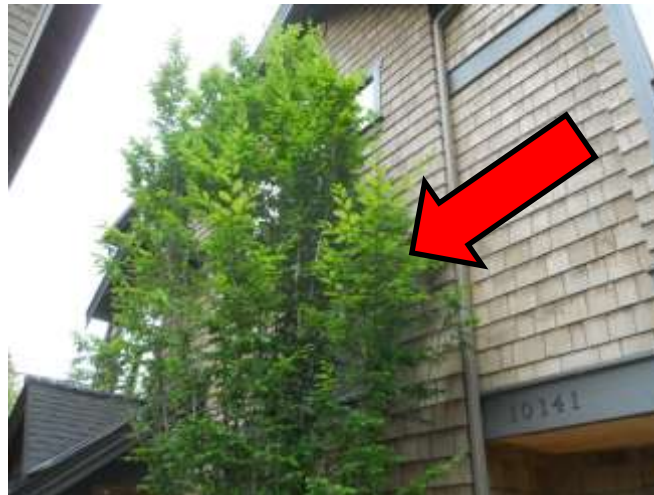
Vegetation in contact with structure WDO conducive condition
