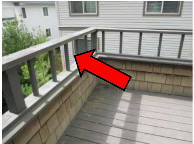
Rails do not appear to comply with code
