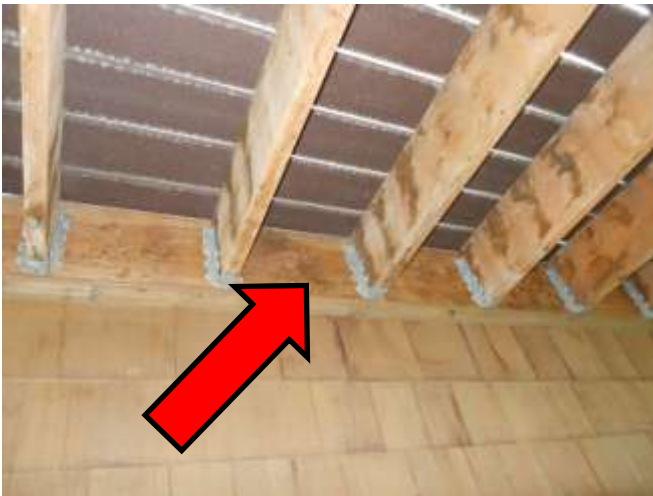
No evidence of lag bolt connection of deck to house
