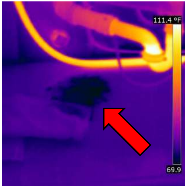
Leak at Kitchen sink
