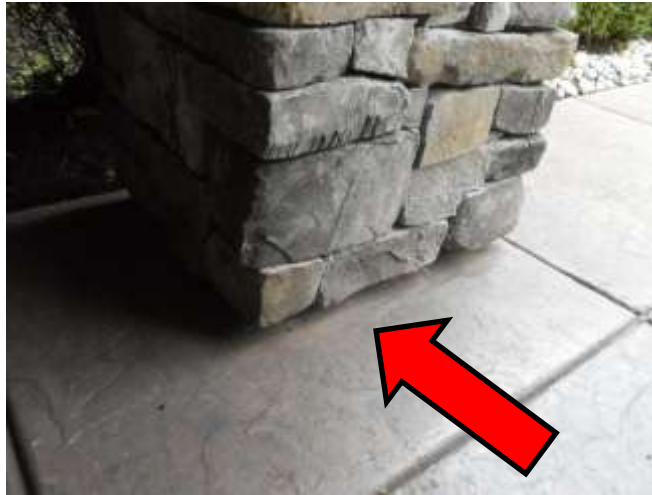
Gap at N.E. patio pier See prior comment in Site section
