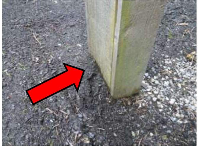
Ground in contact with wood Potential wood rot condition
