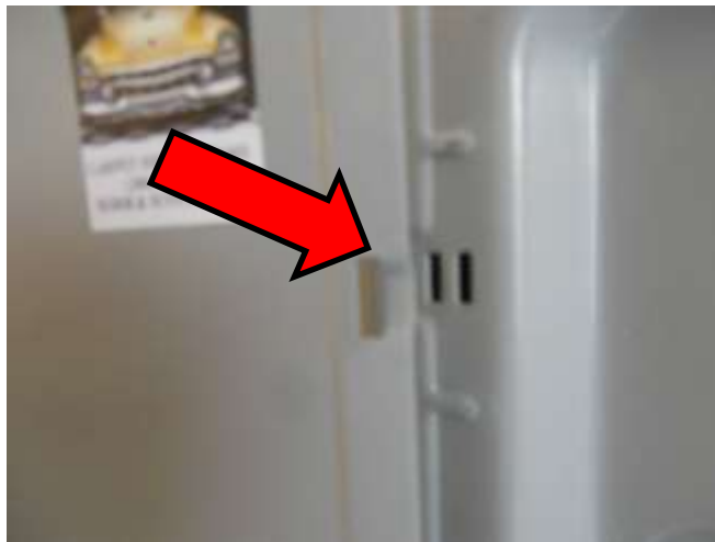
Hinge missing at electrical panel
