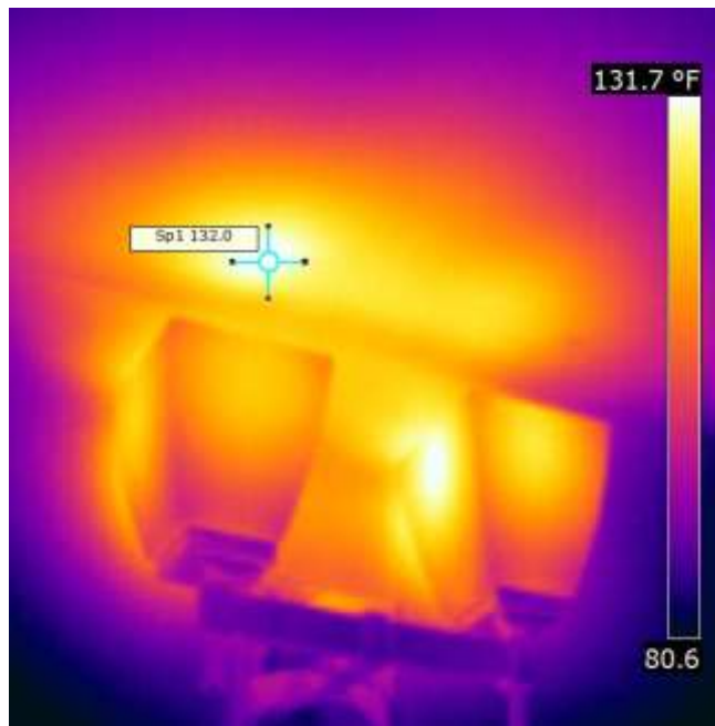
Light fixtures face upwards close to ceiling
