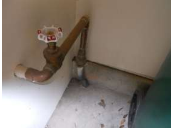
Domestic Water Shut off
