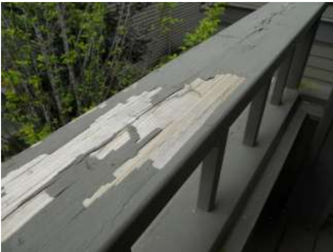
Substantial weathering of deck rails
