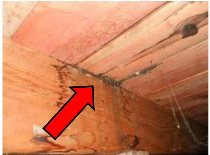
Wood rot at Master Bathroom shower area
