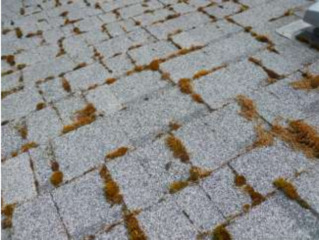
Moss build up
