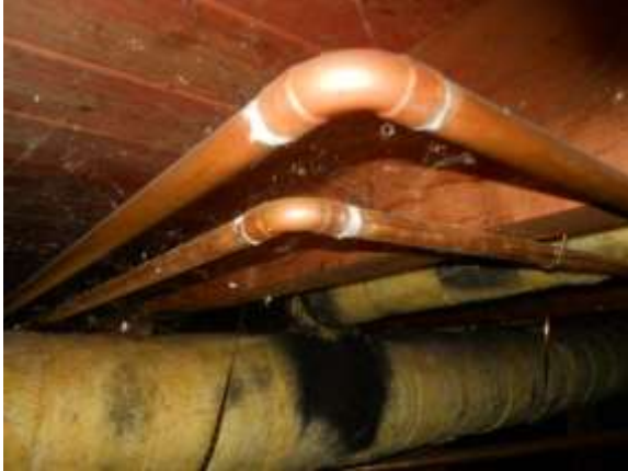
Copper domestic water pipes
