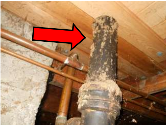
Frass at Master bathroom waste line No ants were visible
