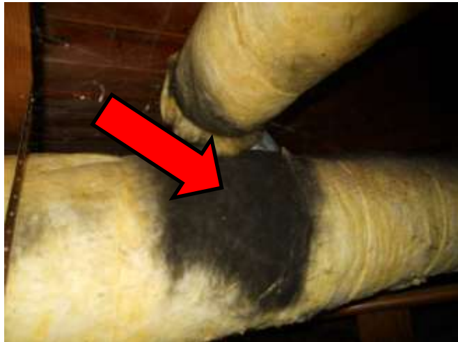
Dark areas indicate air leakage
