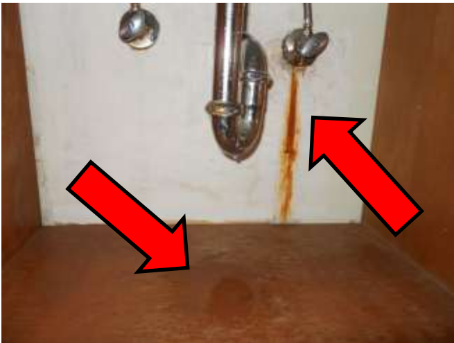
Leaks at bathroom sink and valve
