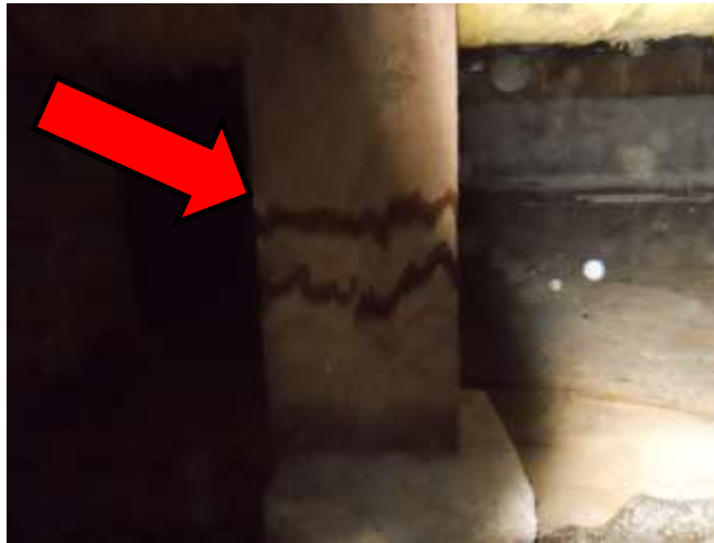
Moisture stains suggest up to 1.5 feet of water in crawlspace
