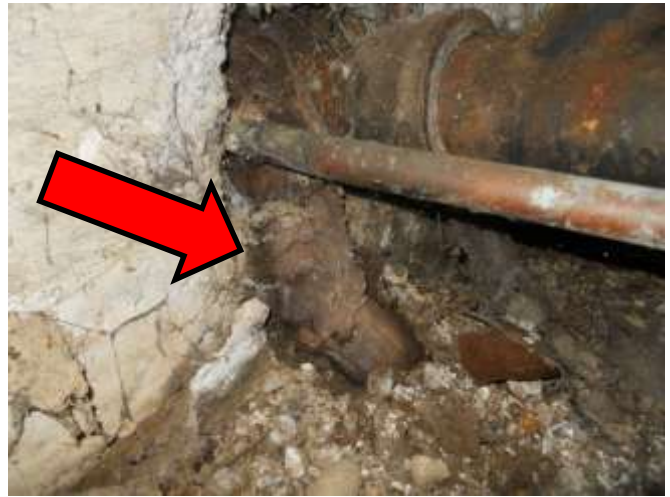
Tree root at entry of plumbing lines
