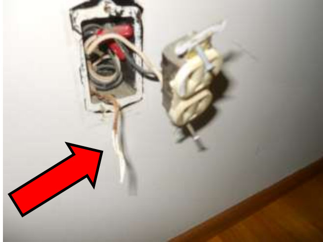
Outlet in bedroom Ground wire not connected to outlet
