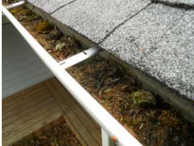
Debris in gutters
