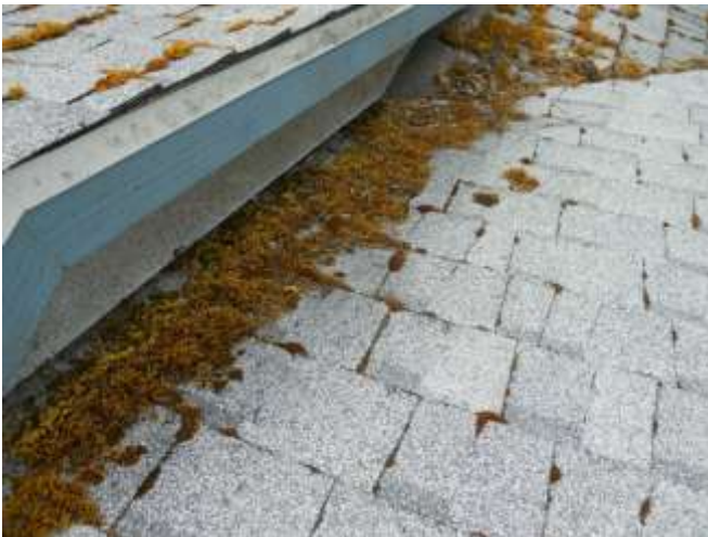
Moss build up
