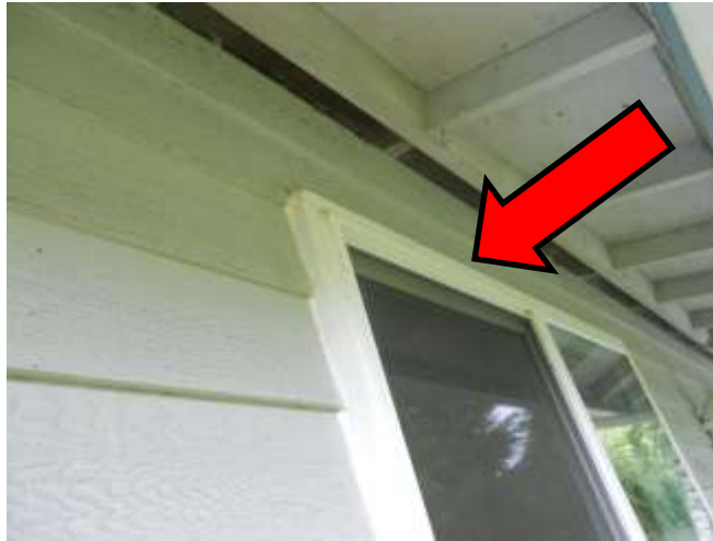
Window trim does not have head flashing
