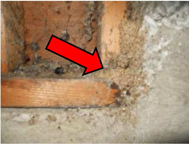
Older frass near foundation crack/stepdown by Master Bedroom
