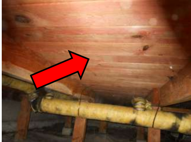
No insulation in crawlspace
