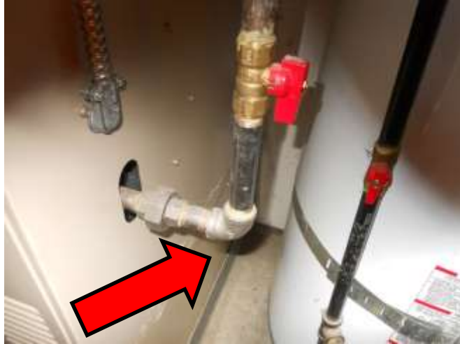
Drip leg not installed at gas piping
