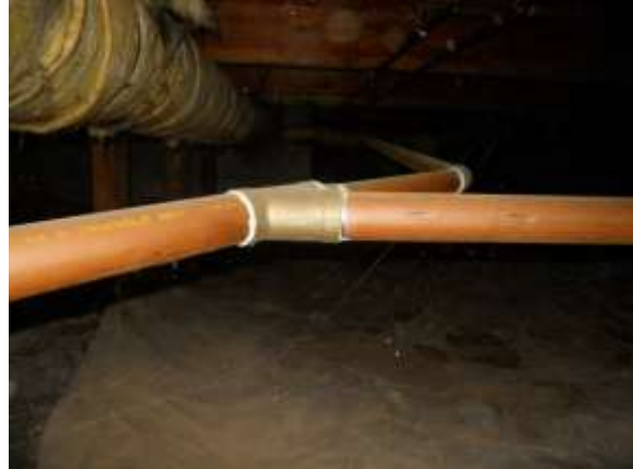
Copper waste lines
