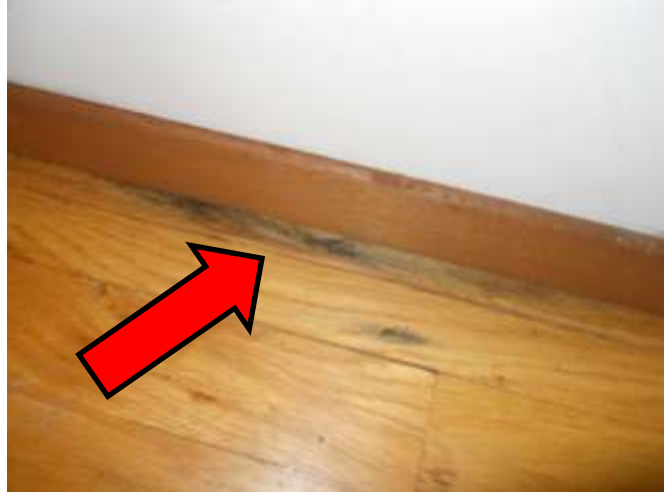
Moisture damage to hardwood adjacent to bathroom
