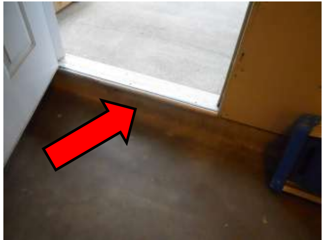
Trip hazard at exterior door
