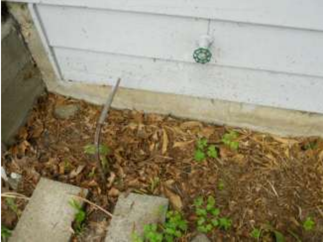
Ground slopes towards house at Master bedroom
