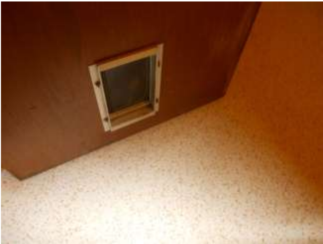
Door to house is not weather-stripped
