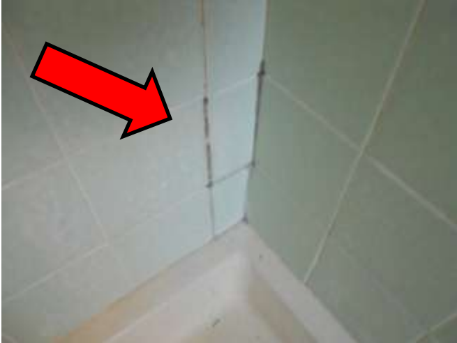
Prior repair to tile in shower
