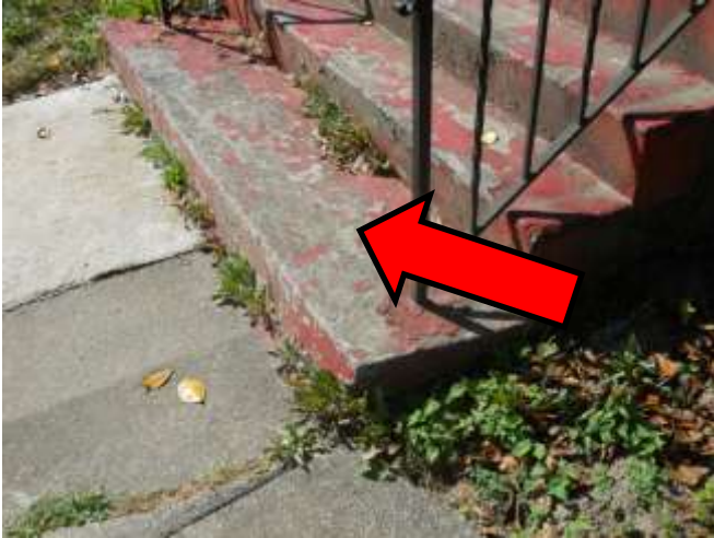
Trip hazard at lower step
