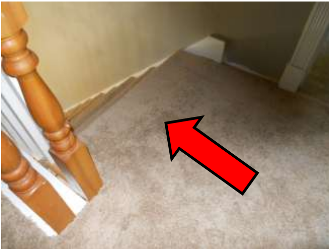
Trip hazard at carpeting tack strip
