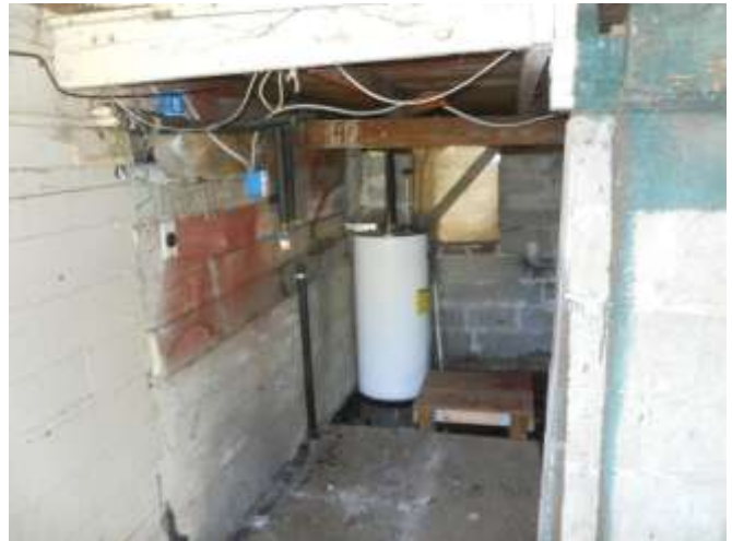
Water heater room should be protected from exterior temperatures (add wall ?)
