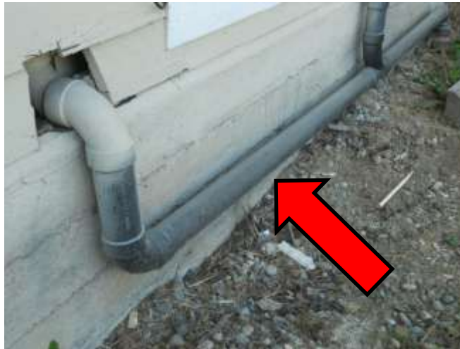
Exposed ABS waste lines
