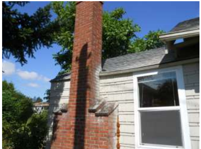
Chimney appears abandoned Cap on top of chimney
