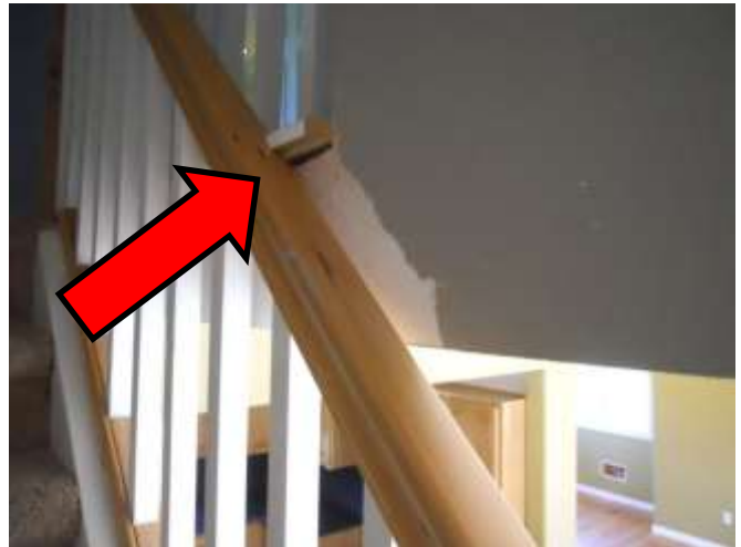
Handrail is not considered "continuous"
