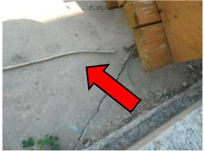
Exposed wire to future garage
