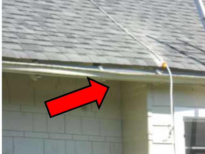
Bent gutter (typical)
