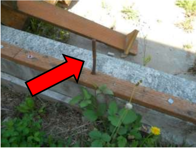
Safety hazard at foundation bolts
