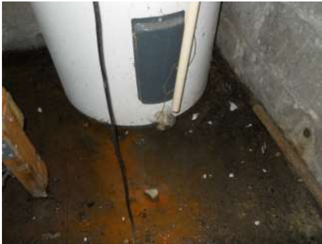
Moisture beneath water heater
