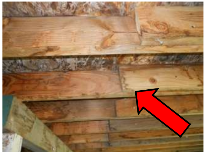
Joists are spliced but not supported
