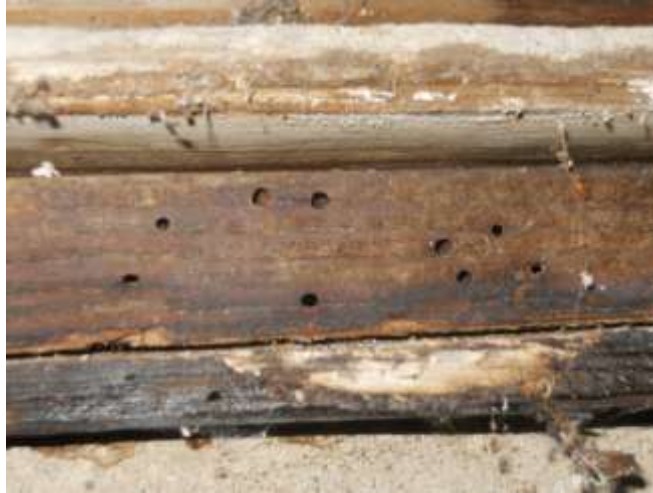
Beetle emergence holes at rear mudsill
