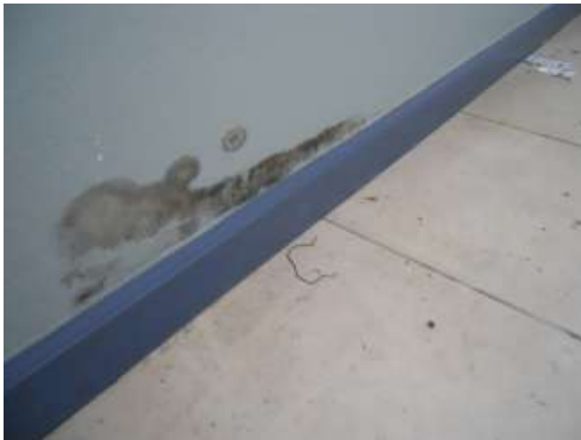
Mold like substance at wall
