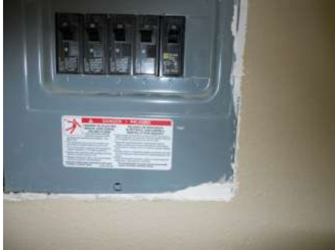
Unable to open sub panel cover
