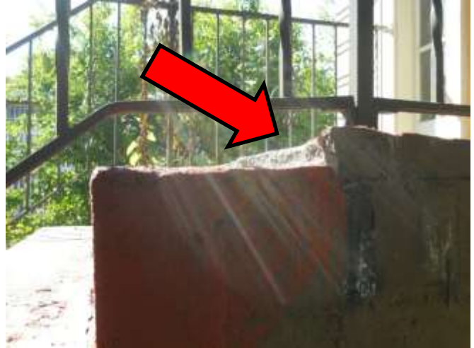
Trip hazard at upper step
