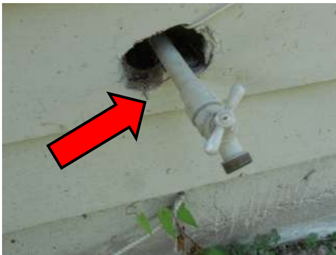
Substantial gap at siding
