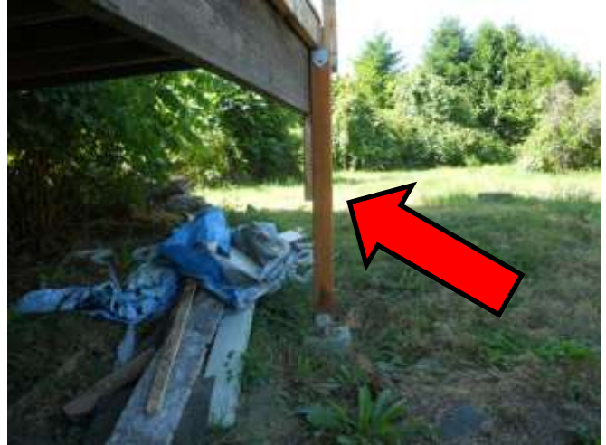
Post out of plumb and not secured
