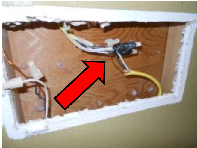
Wire splice at Living Room heater space does not appear to meet electrical code (should be in junction box)
