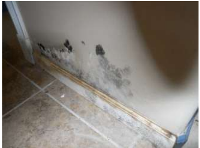
Mold like substance at wall
