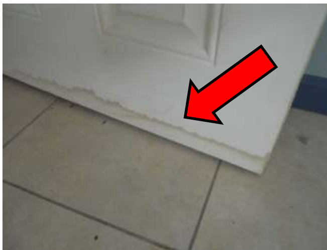
Moisture stains at base of door
