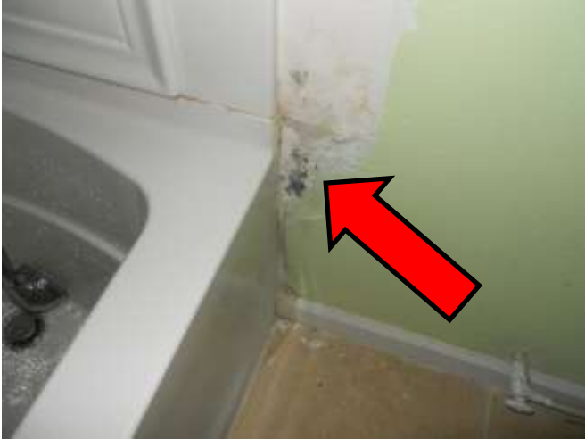
Moisture damage at shower wall
