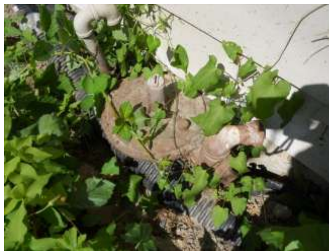
Gas valve located at side yard Appears inoperative Call for locates prior to any side yard excavation !
