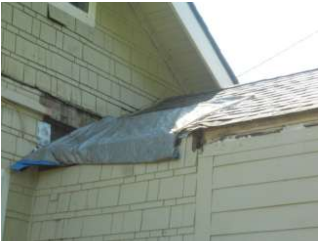
Tarp and missing siding at Master Bedroom
