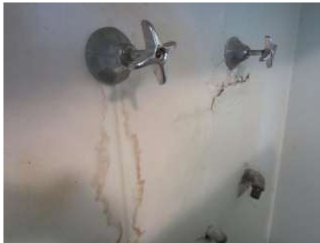
Moisture stains at washing machine valves
