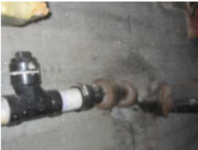
(3) types of plumbing waste pies
