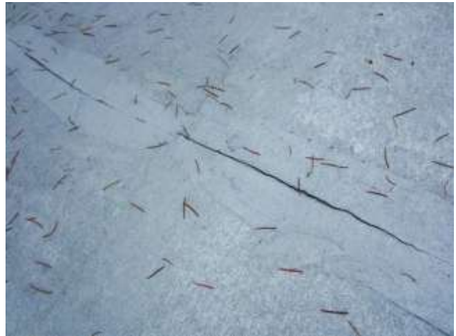
Crack and prior patch at rear area above Master Bedroom
