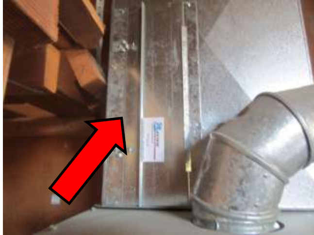
Furnace filter compartment
