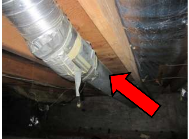
Un-insulated heating duct
