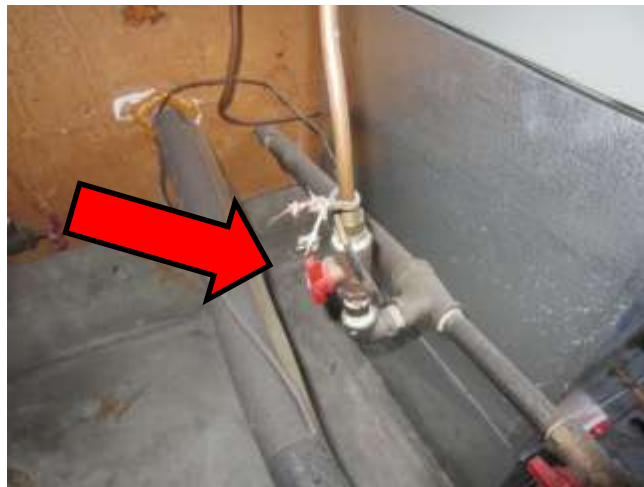
Gas shut off for fireplace is located in garage
