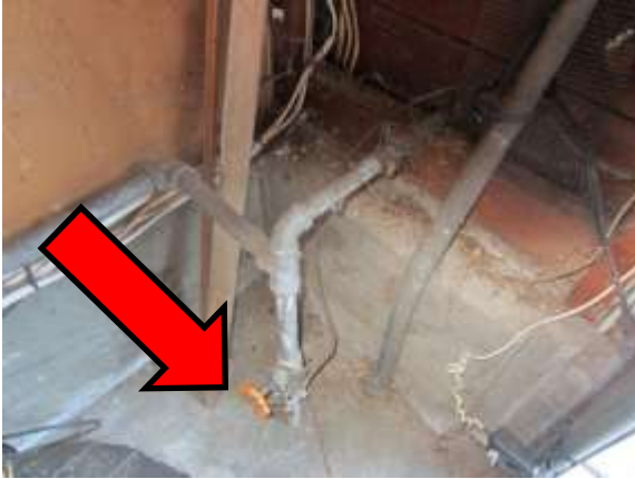
Domestic Water Shut off
