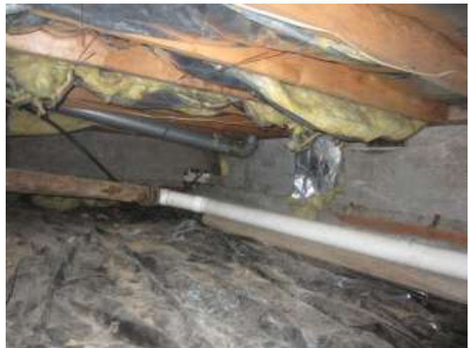
Sewer discharge pipe in not properly supported Support is from a wood member below
