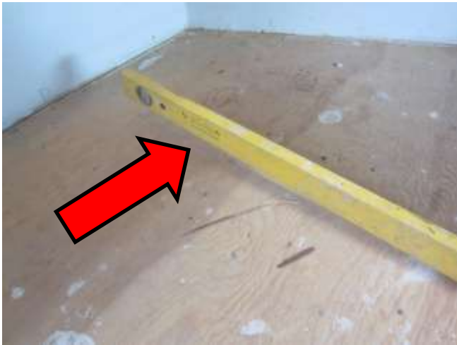
Floor height inconsistency is greater than 1"
