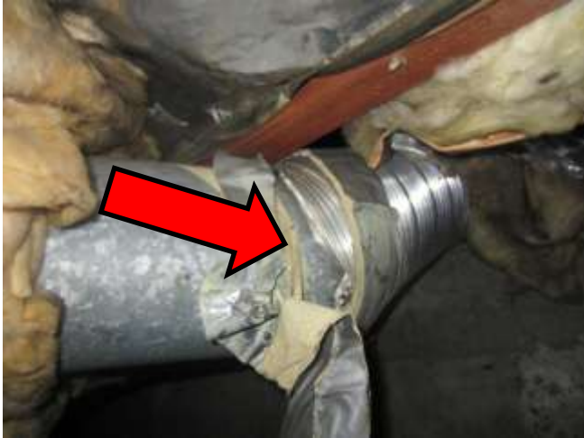
Leakage at heating duct
