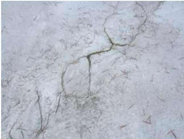
Cracks at valley
