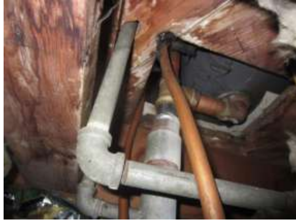
Copper and galvanized supply pipes
