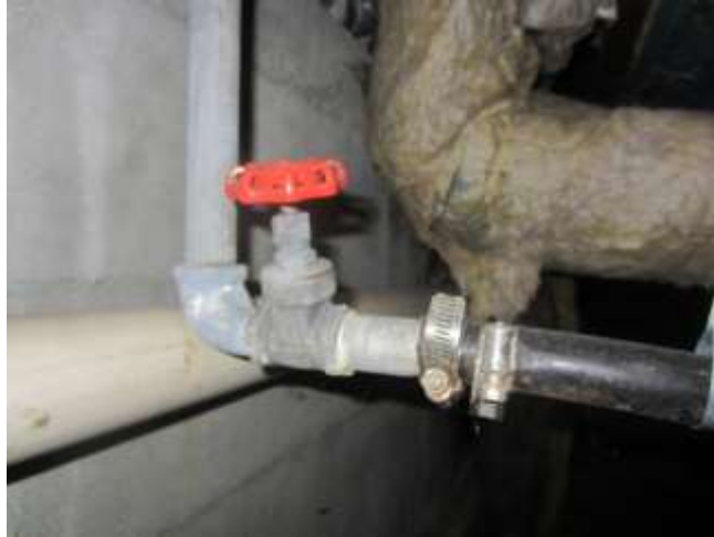
Valve to poly pipe near rear foundation wall Presumed to be for rear yard hose
