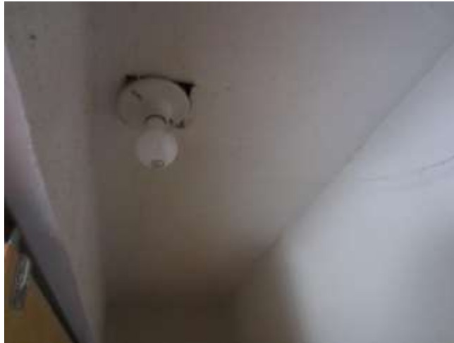
Fire hazard from exposed bulb
