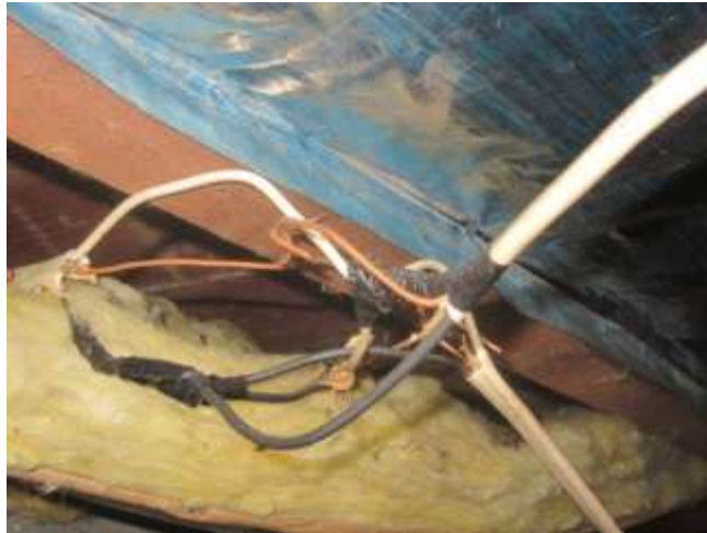
Improper wire splice
