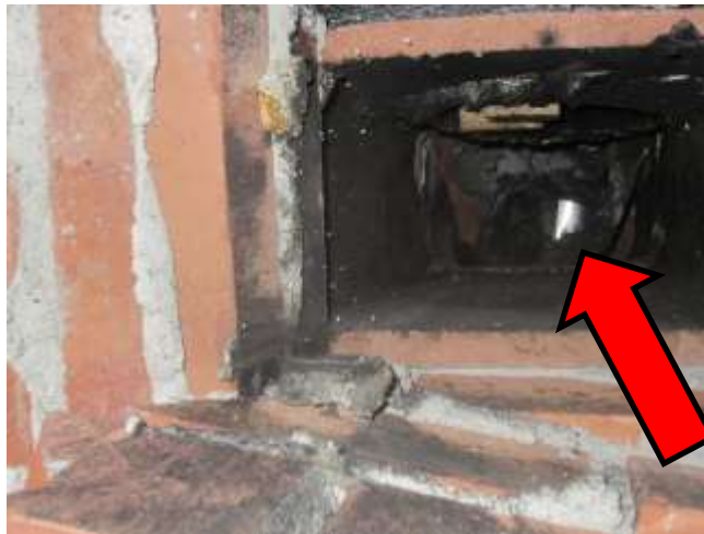
Furnace flue discharges into chimney Chimney is lined where visible
