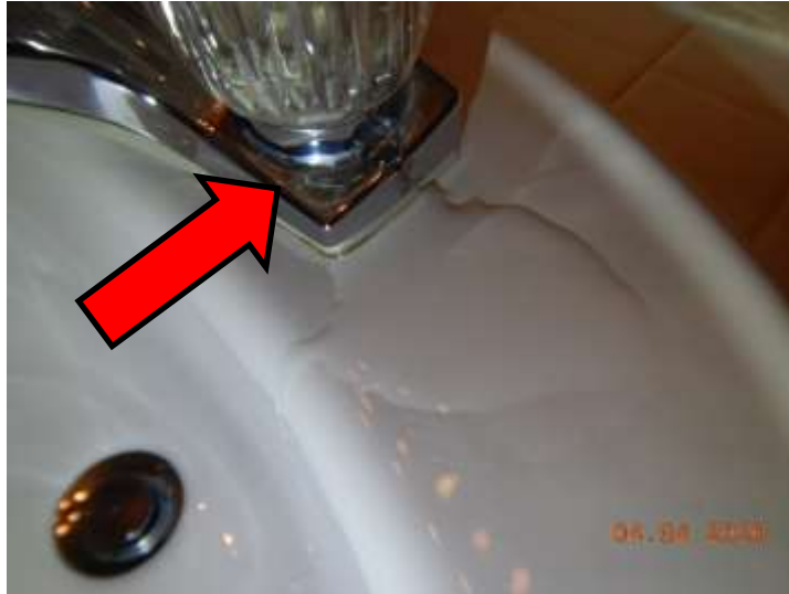
Leakage from the cold water valve
