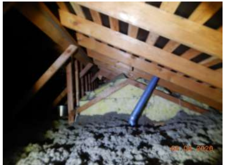
Laundry room vent
