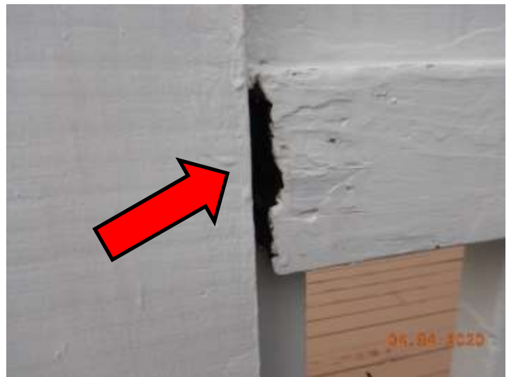
Evidence of wood rot
