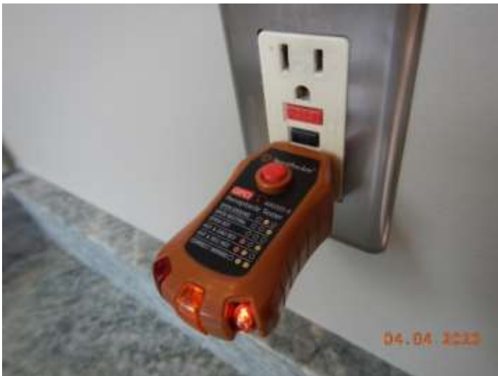
This outlet does not trip when tested
