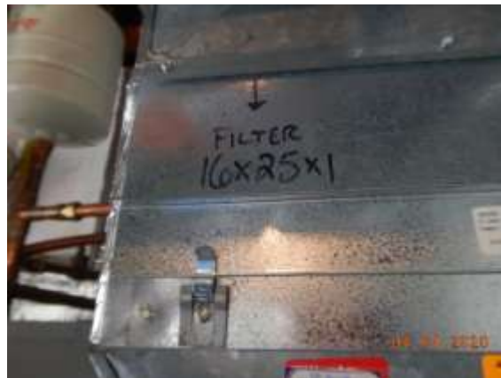
Furnace filter location
