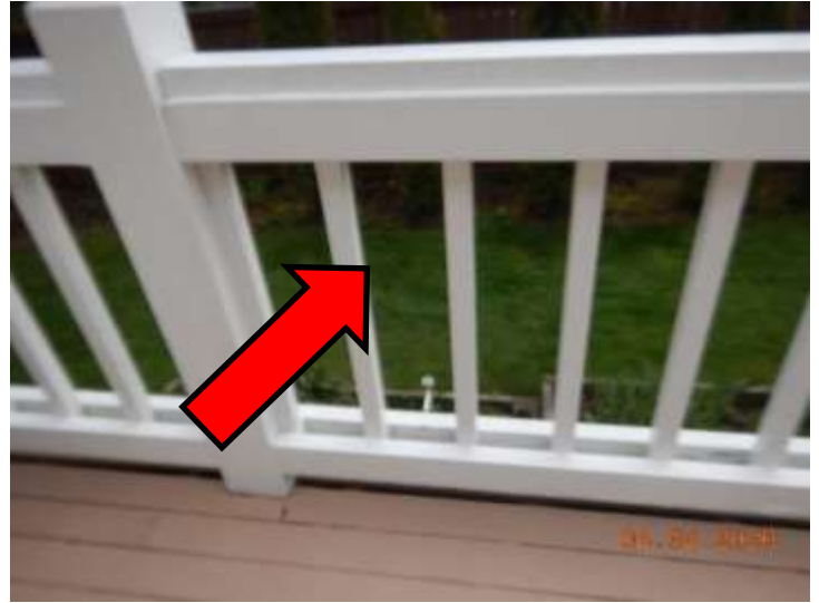
The spacing at the barricade exceeds 4"
