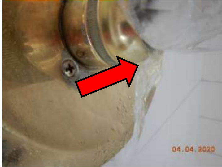
Leakage from the shower valve when active
