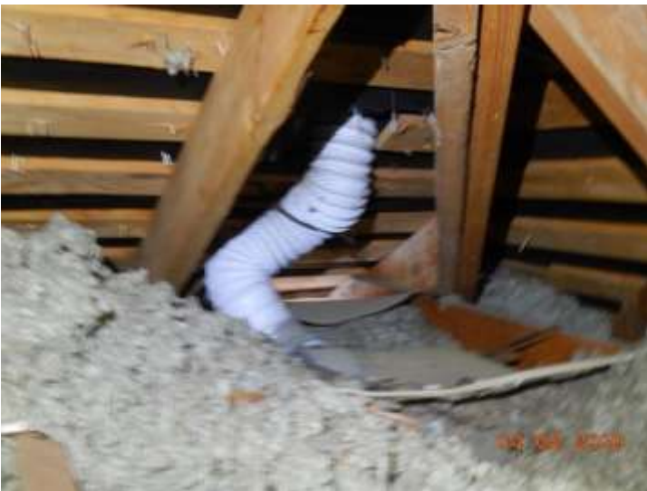
Bathroom ventilation duct (typical)
