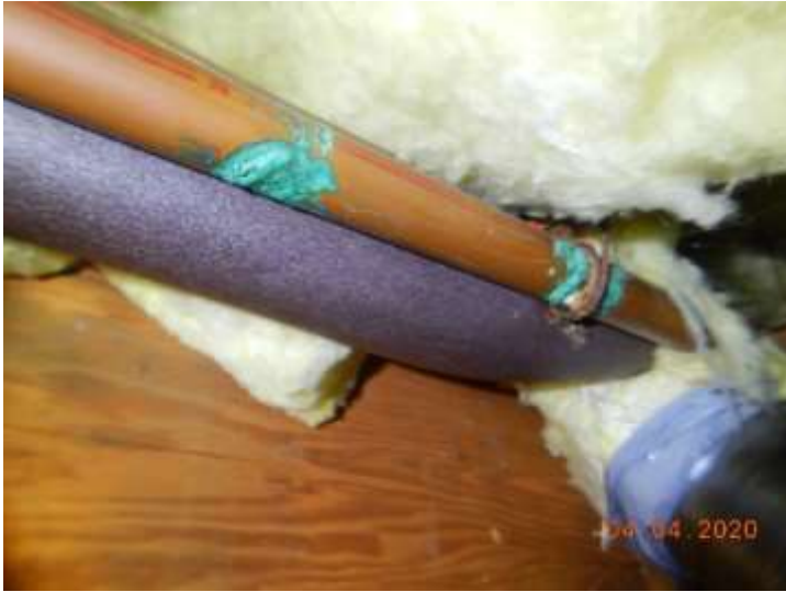
Domestic water supply pipe
