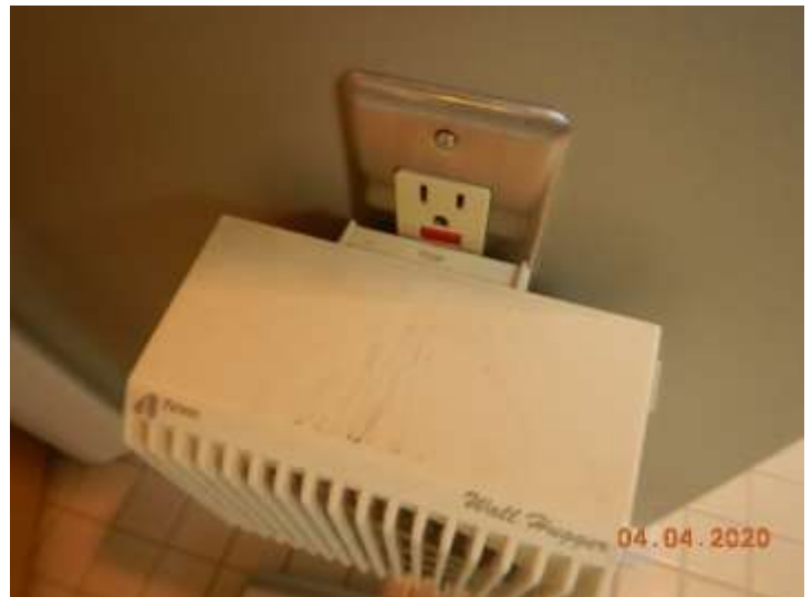
The tub motor is properly GFCI protected by this outlet
