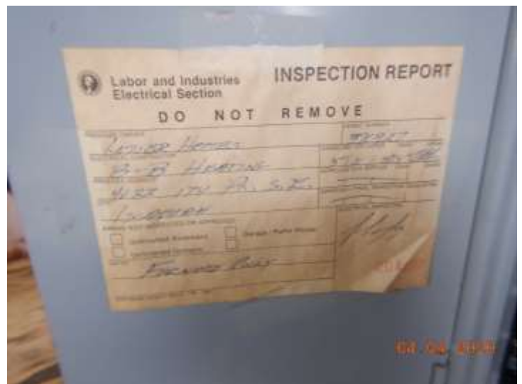
Electric service permit tag
