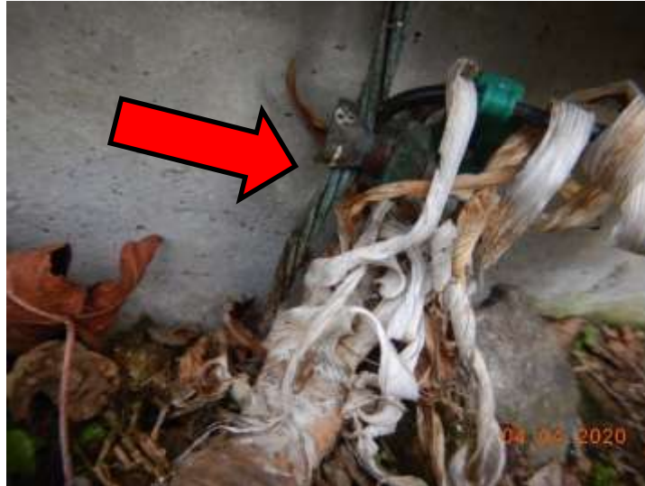
Electricval system grounsing
