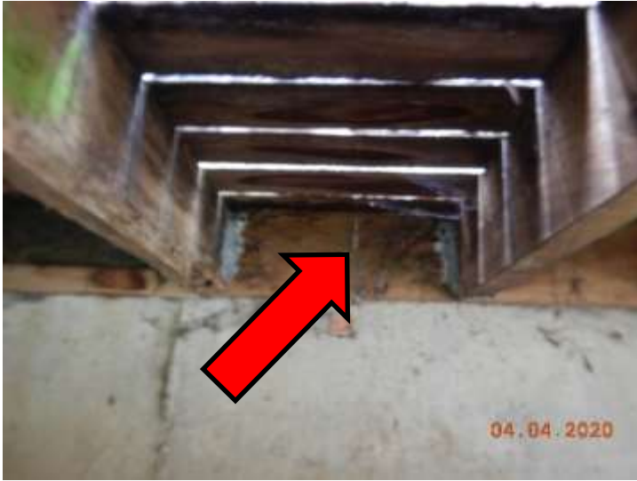
Lag bolts were not visible
