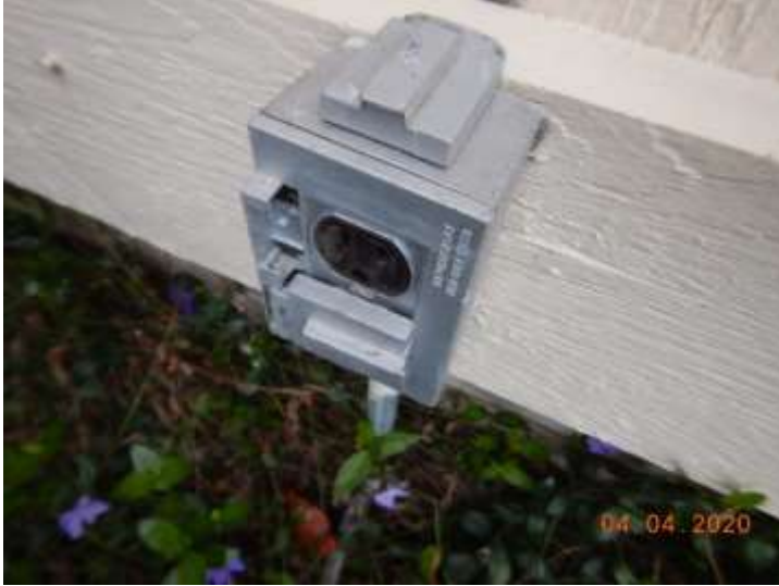
Missing weatherproof cover
