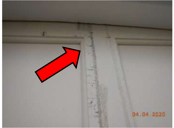
Evidence that the West door is rubbing on the door frame or mechanism
