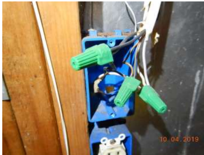
Improper wire splice
