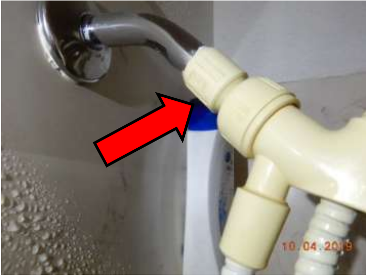
Leakage from the shower head connection
