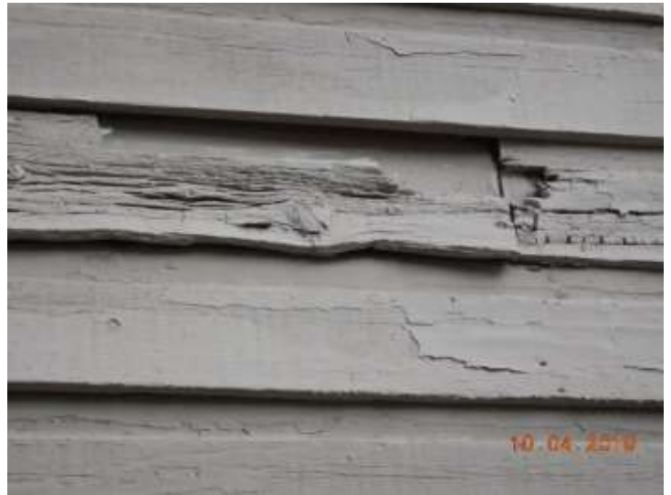
Deteriorated siding at the South facade
