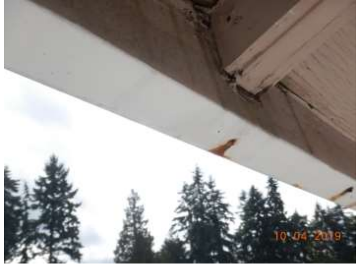
Rust drips areas at the front upper gutter
