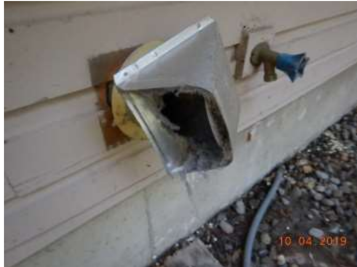
Improperly positioned dryer vent
