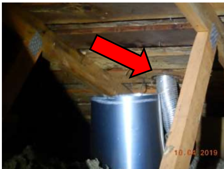
Bathroom ventilation duct
