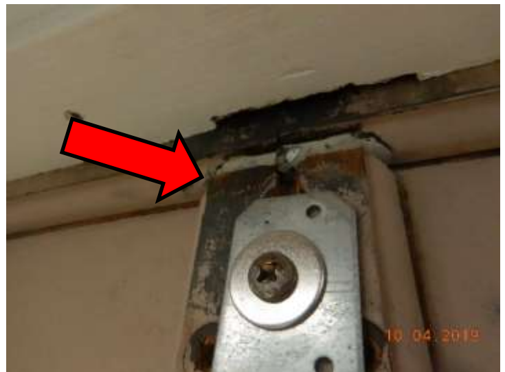
Prior repairs to the failing upper panel
