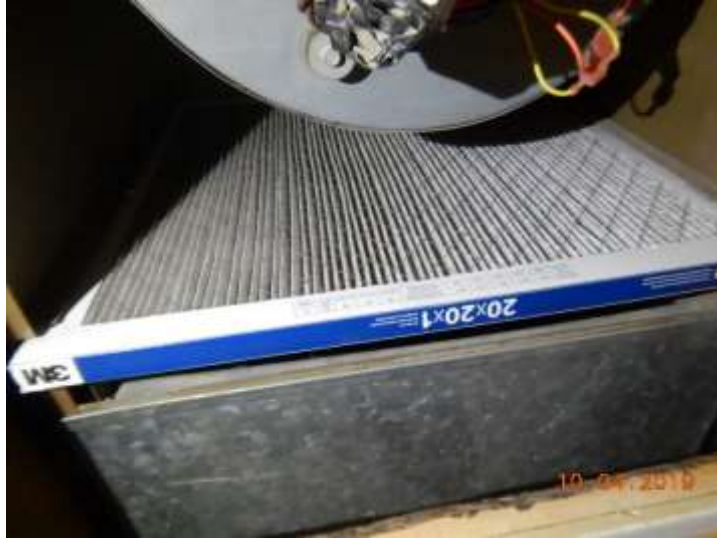
Furnace filter location
