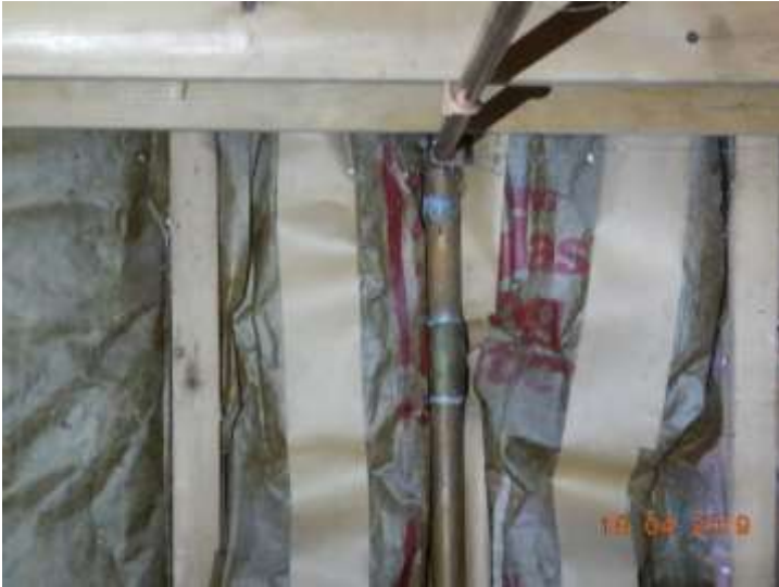
A domestic water shut off valve MAY be located on the other side of the crawlspace in the occupied garage
