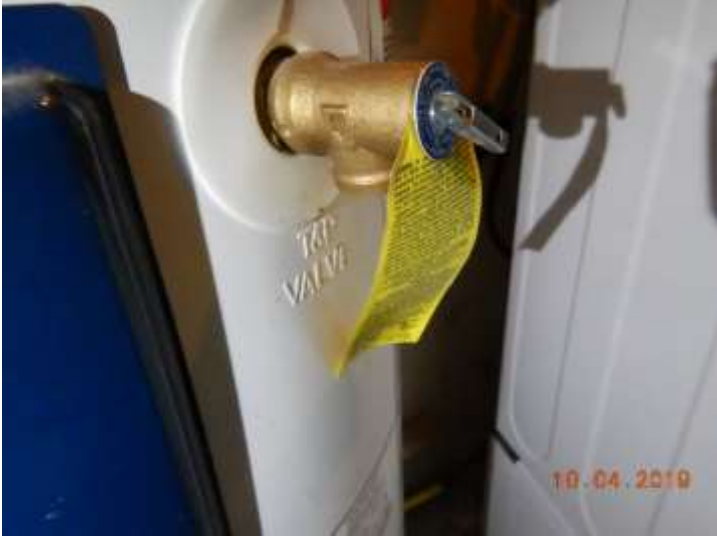
There is no extension on the TPR valve
