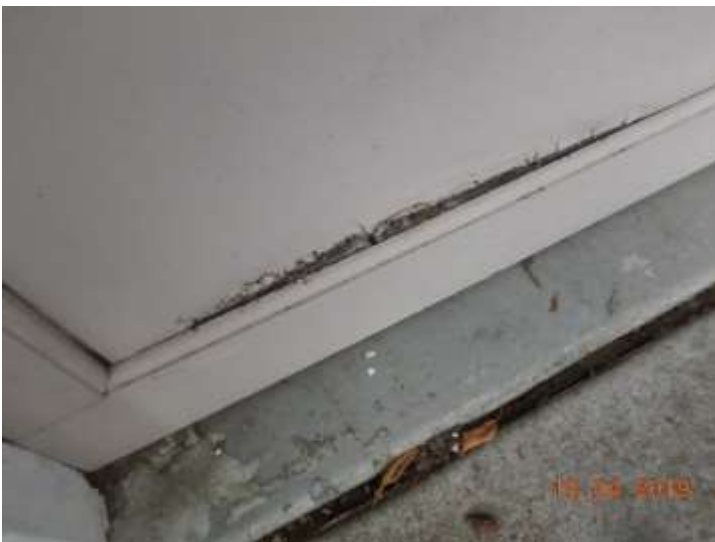
Deteriorated garage door panel
