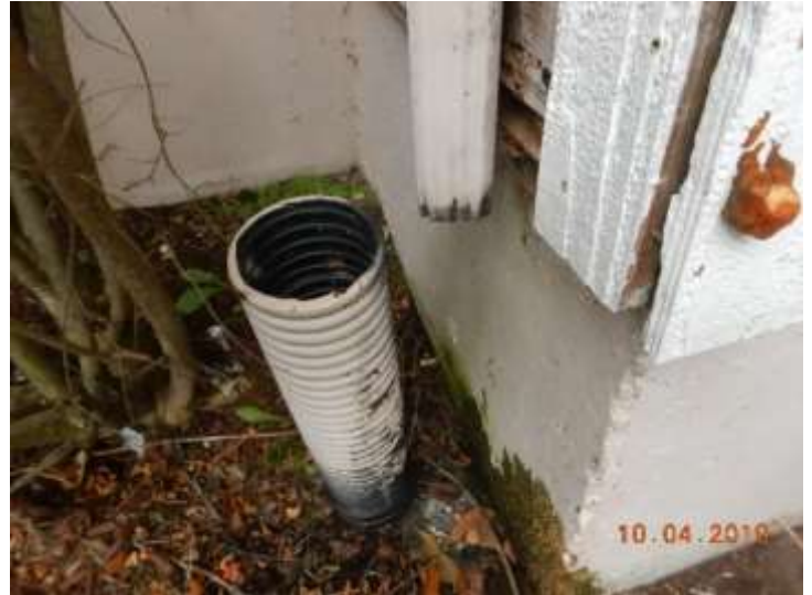
Downspout connection not aligned (WDO conducive condition)
