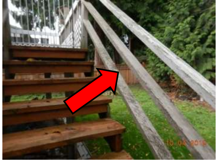
The barricade is unstable and is leaning
