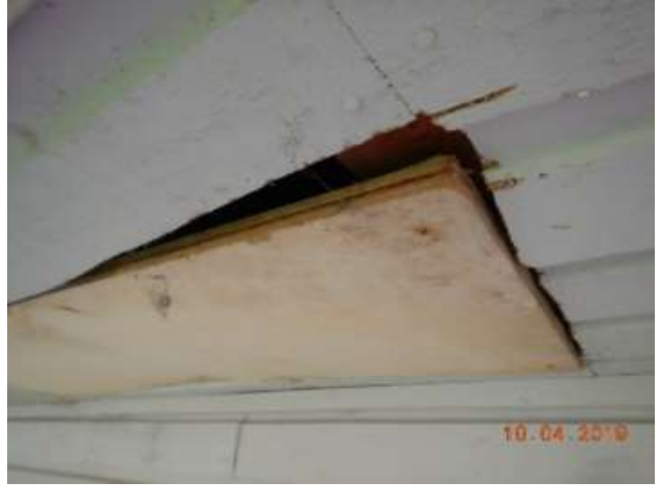
Gaps at the soffit
