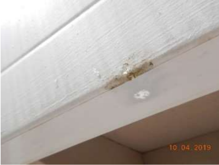
Hole in a gutter. Tape is placed over the hole to attempt to stop leakage
