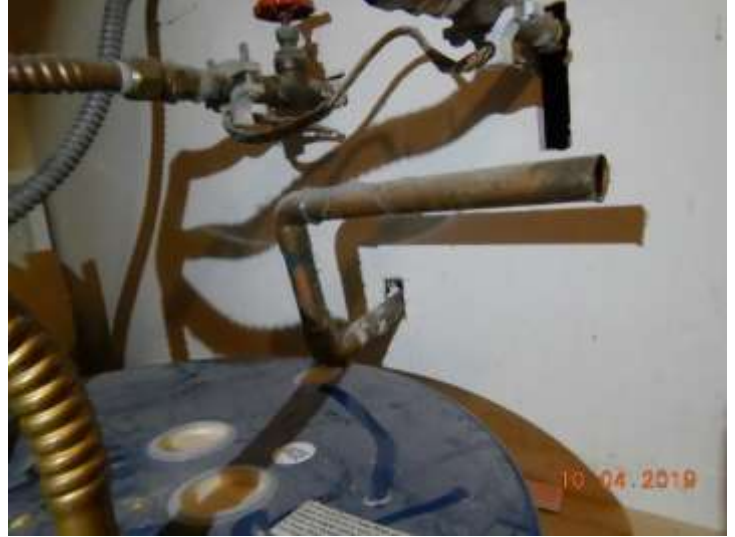
Connection for the TPV valve (not used)
