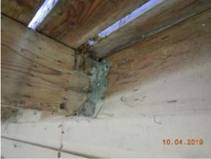
The deck is not lag bolted to the home
