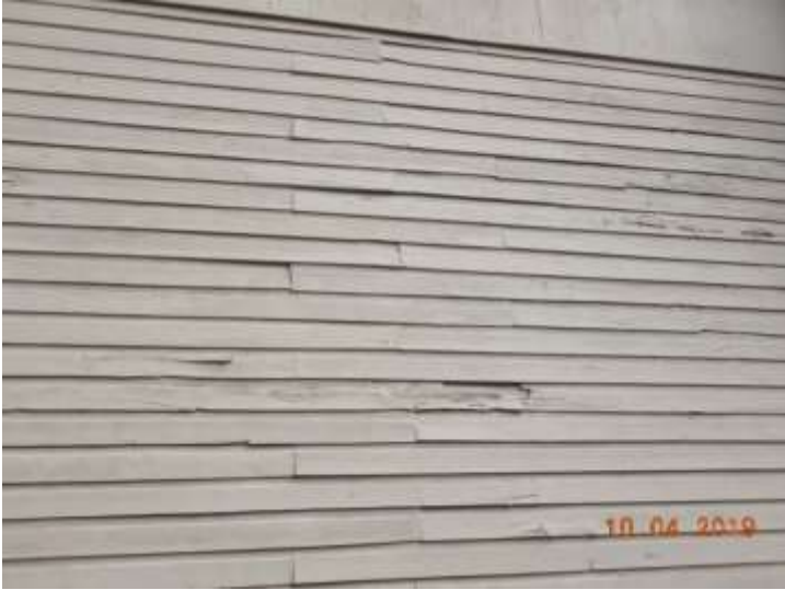
Deteriorated siding at the South facade
