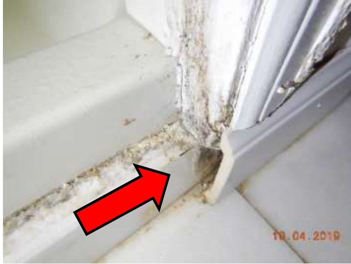
Moisture related damage to the baseboards and trim
