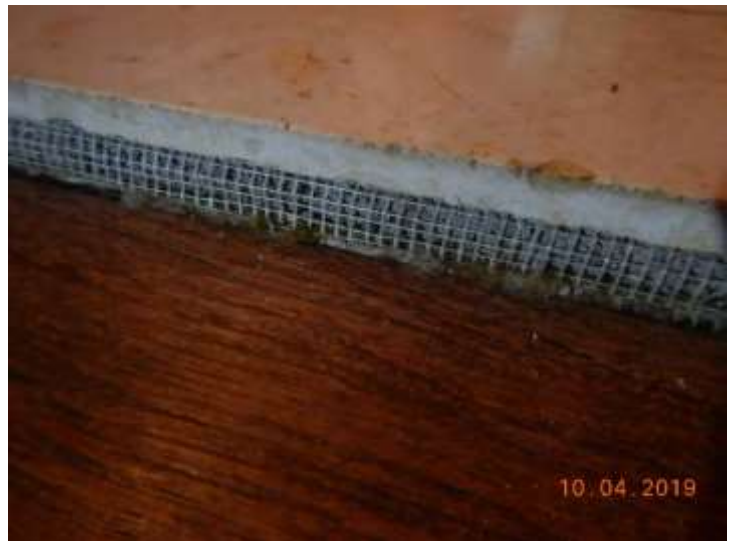
Large vertical height difference @ main bathroom
