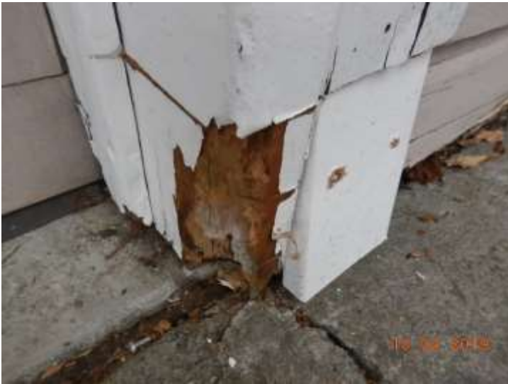
Deterioration of the garage door center divider
