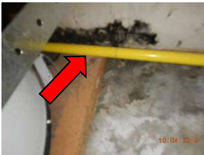
Evidence of black mold
