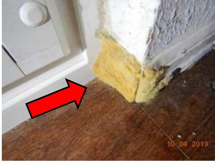
Moisture damaged baseboards
