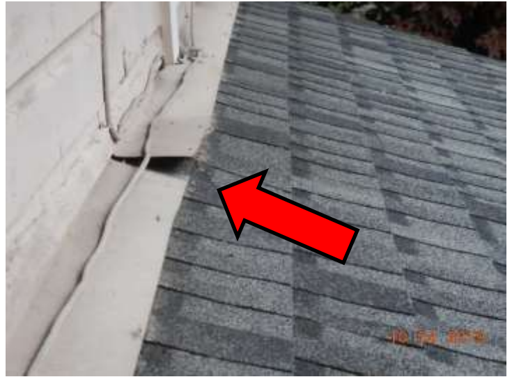
Front roof. The roof to wall metal should be secured to lay flat
