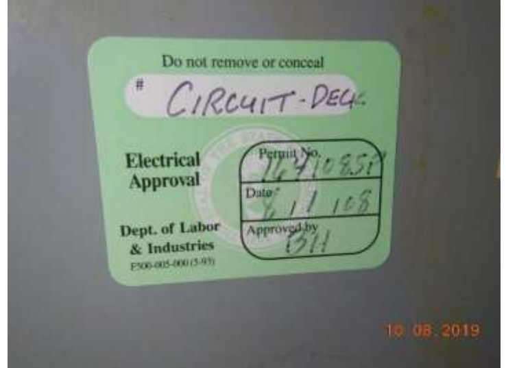
Electric service permit tag
