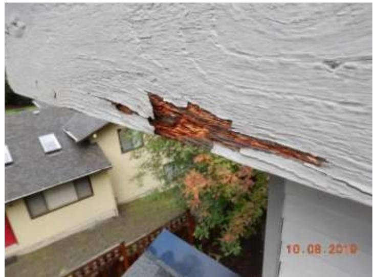
Deterioration of a fascia board
