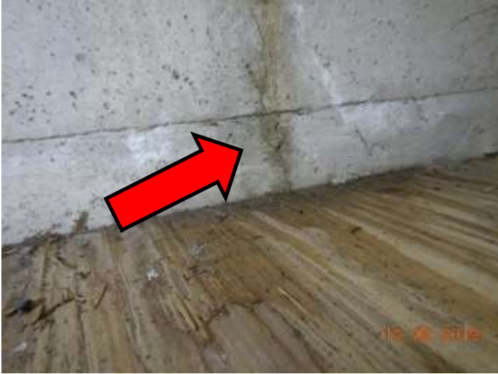
Moisture at the workspace
