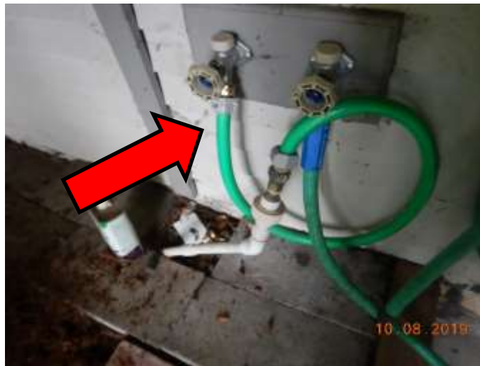
Connection to a hose bib
