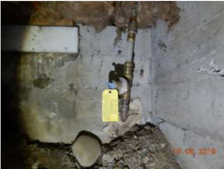
Domestic water pressure reducing valve
