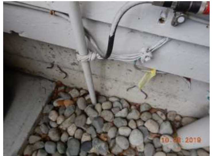
Electrical system grounding
