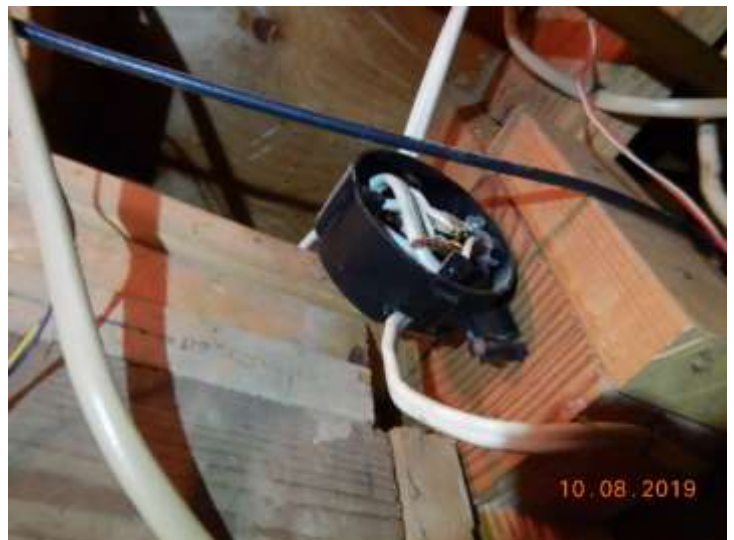
Open junction box
