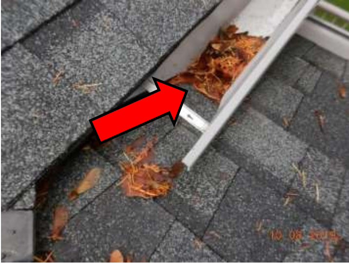
Gutter clogged with debris
