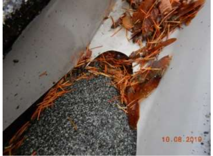
The hole at the end of the gutter is very small (the debris was pulled back by inspector)
