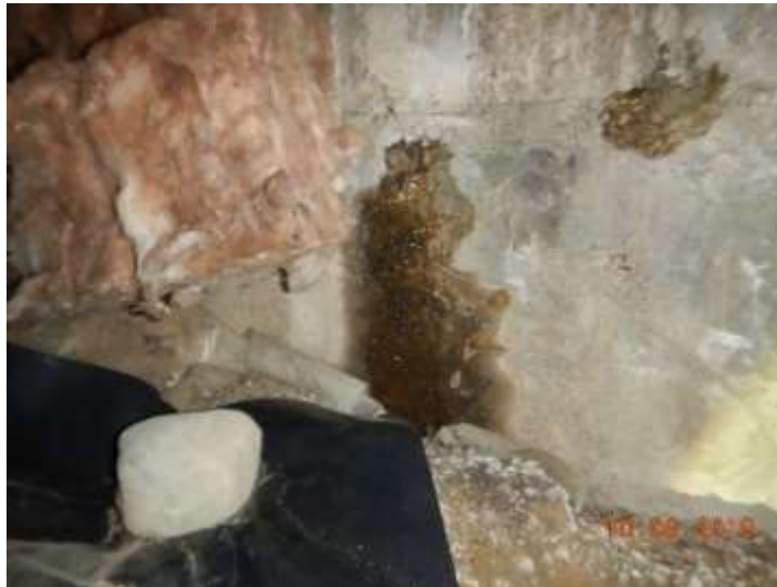
Moisture at the crawlspace
