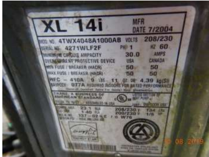
The heat pump is dated 2004
