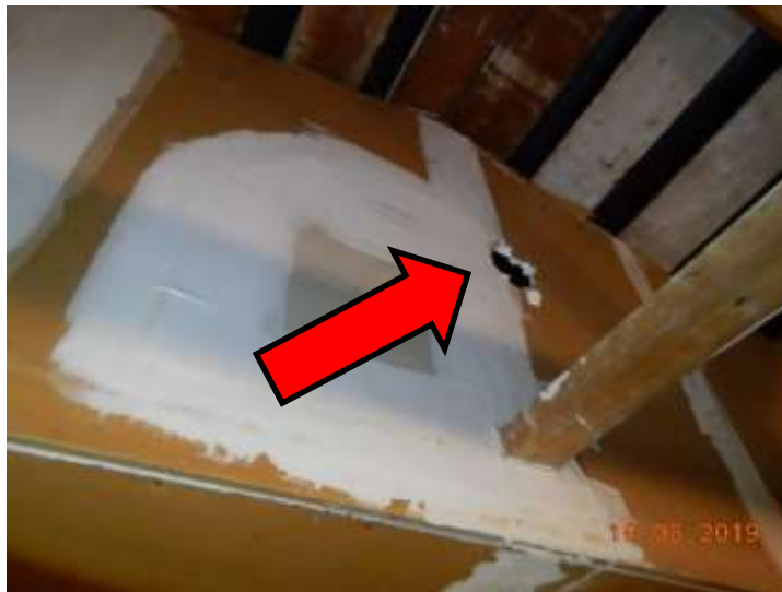
Hole in the drywall
