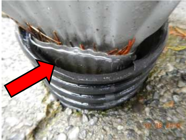
Standing water in the pipe after the recent rainfall
