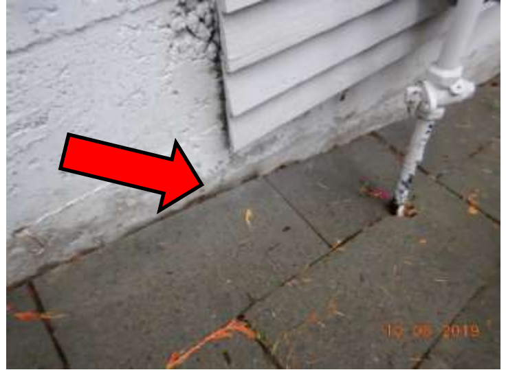
Aproximate location of the moisture intrusion
