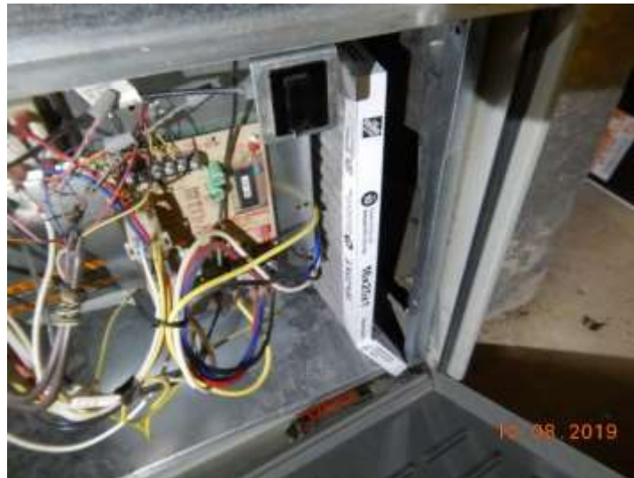
Furnace filter location
