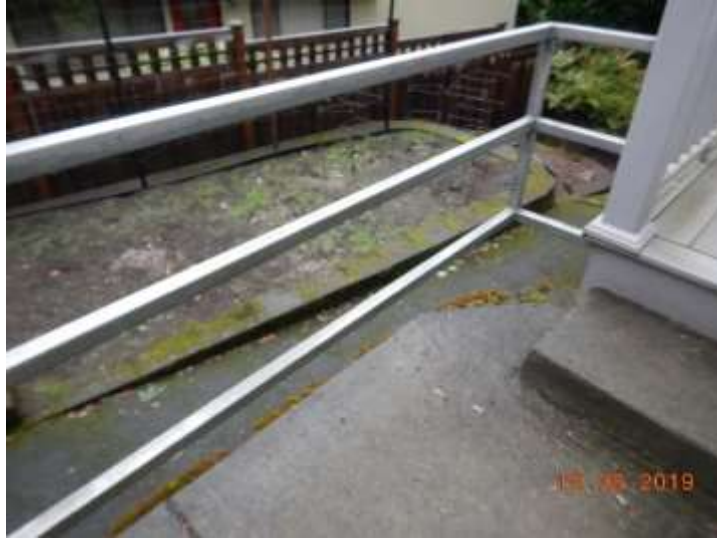
Baluster spacing exceeds 4"
