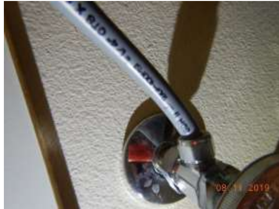
Polybutylene pipe @ sinks
