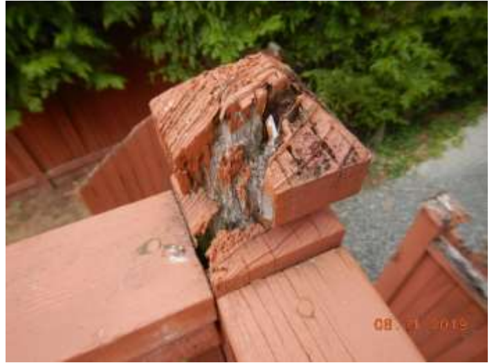
Rotting barricade post (typical)
