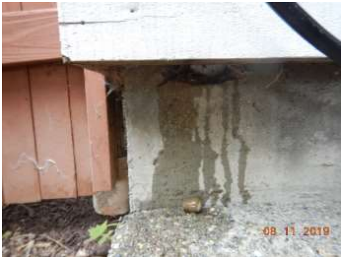
Water running from the siding at the rear hose bib
