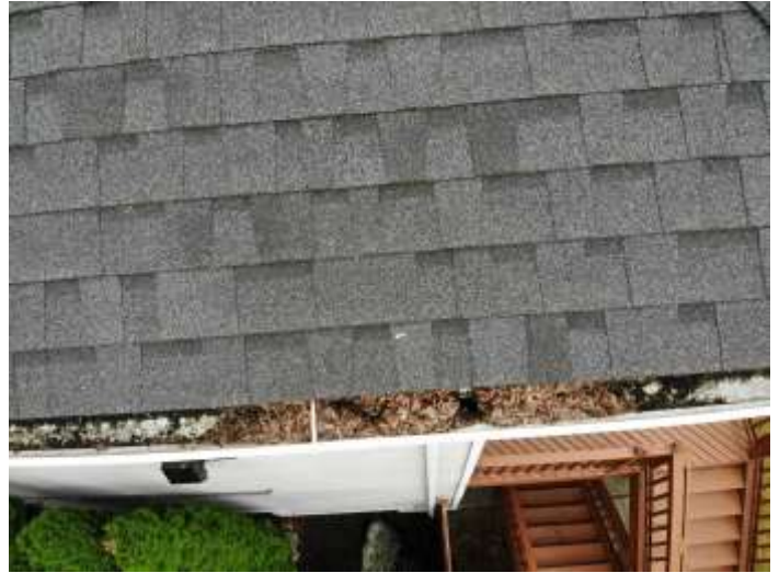
Debris at an upper rear gutter
