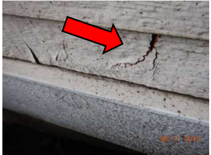
Failed siding at the Living room area
