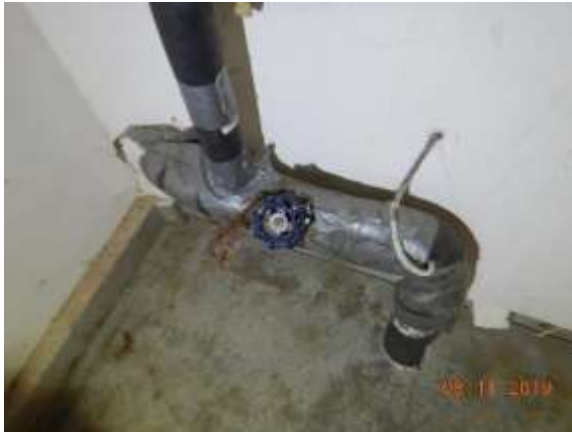
Domestic Water Shut off
