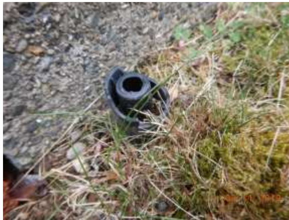
Damaged irrigation head
