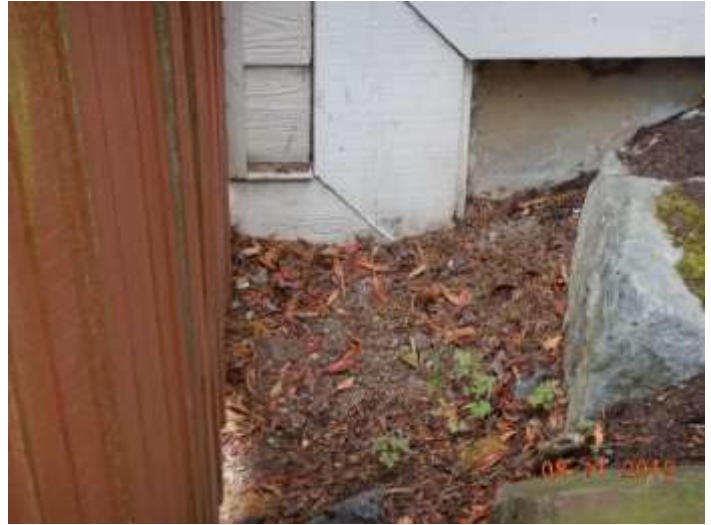
Ground in contact with the siding (WDO conducive condition)
