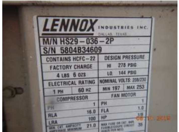
The compressor appears to be dated 2004
