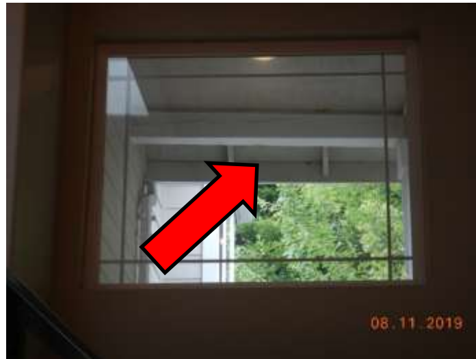
Evidence of settlement (sloping beam)
