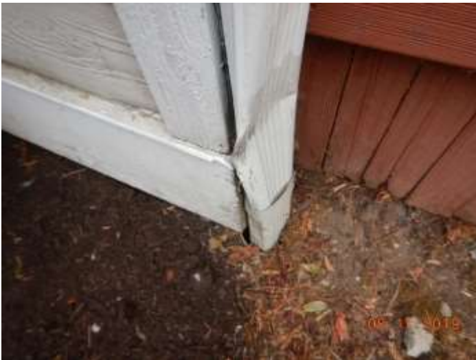
A downspout at the rear of the home is crushed, however appears to service its intended purpose
