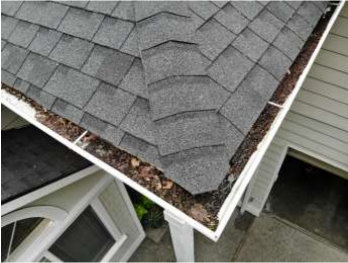
Debris in the gutter above the entryway
