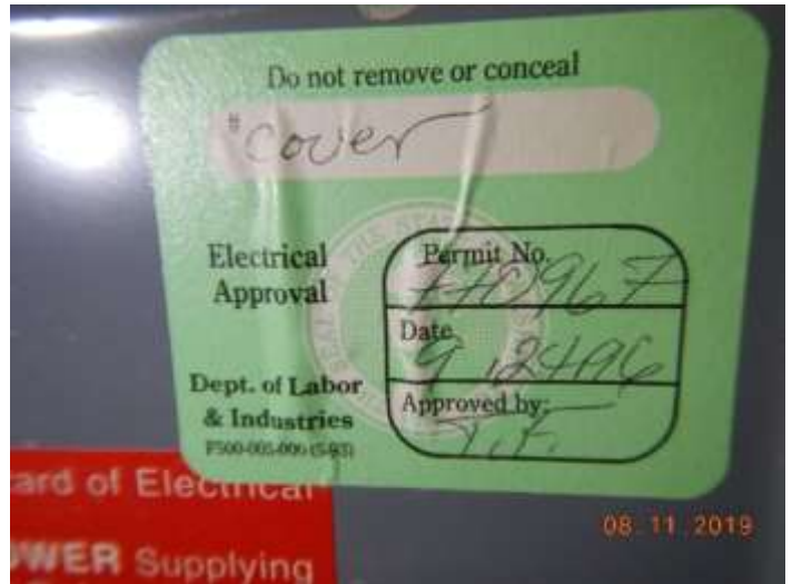
Electric service permit tag
