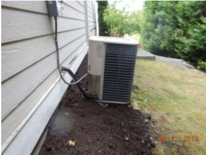
The compressor is not level
