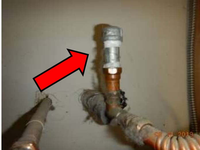
Appears that an expansion tank was removed from this location above the water heater
