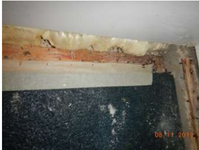
Settlement of 2" +/-; expansion foam has been added. The carpeting was unsecured at the outer corner of the room
