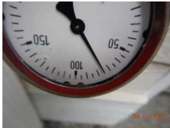
Water pressure is adequate and not excessive
