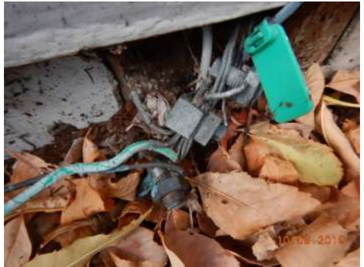
Electrical system grounding
