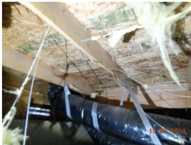
Missing under-floor insulation
