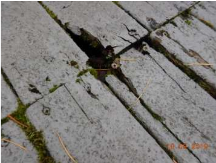
Wood rot at the decking
