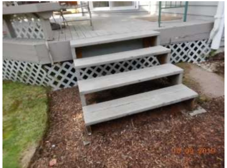
A graspable handrail should be installed where there are 4 or more risers
