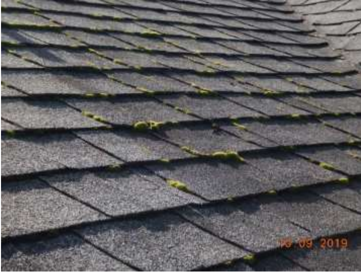
Minor moss on the roof
