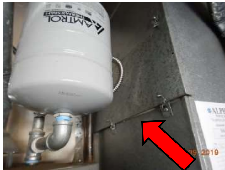
The furnace filter access appears to be partially blocked
