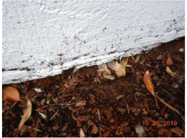
Wood rot at the band board near the entryway
