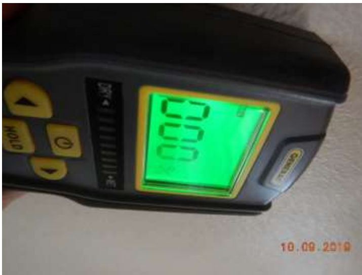
There was no moisture indicated at the cold spot
