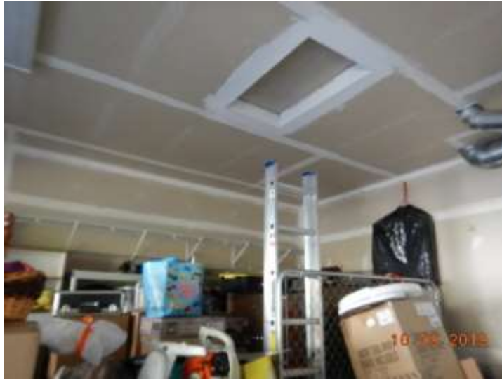
No access to the garage area attic
