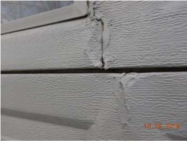
Metal fatigue cracks
