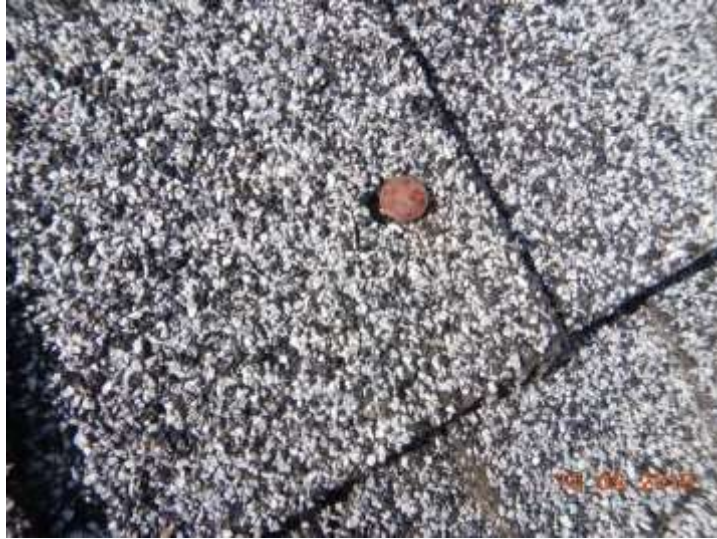
Exposed nail head
