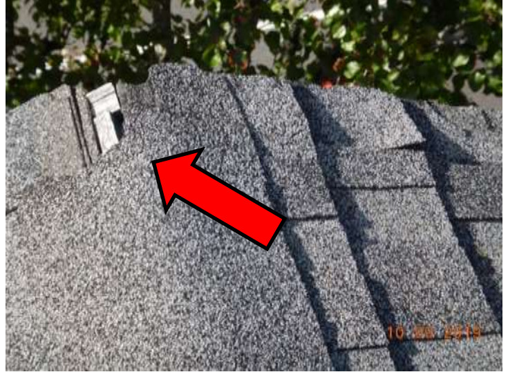
Wind related damage
