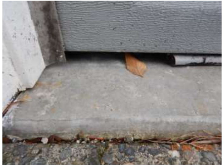
The gap at the weather-stripping may allow pest intrusion
