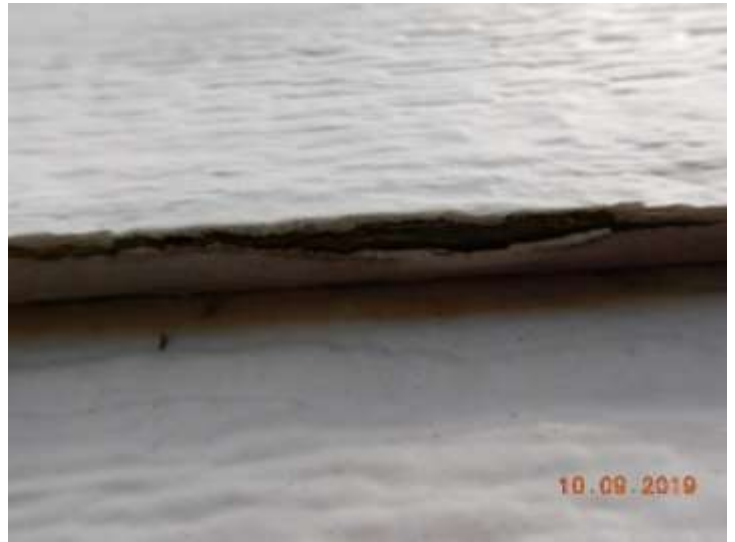
Failed lower edge of a siding board
