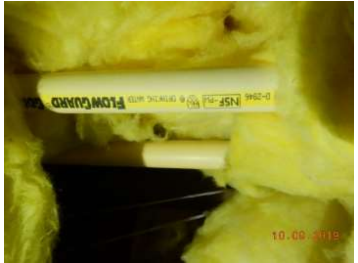
CPVC domestic water distribution pipes
