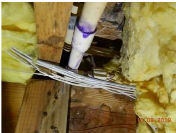
Evidence of a prior repair or modification to the plumbing pipes. See the comment in the Plumbing section regarding CPVC piping
