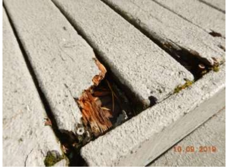
Wood rot at the decking
