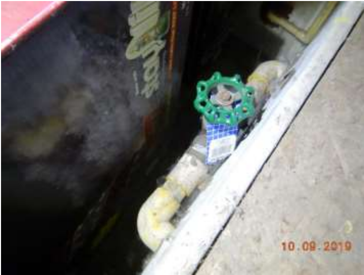
Domestic water shut off
