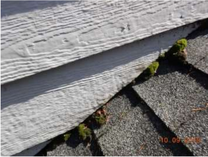
The lower edge of the siding at the rake wall is very brittle
