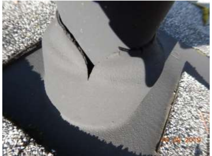
Cracked plumbing vent
