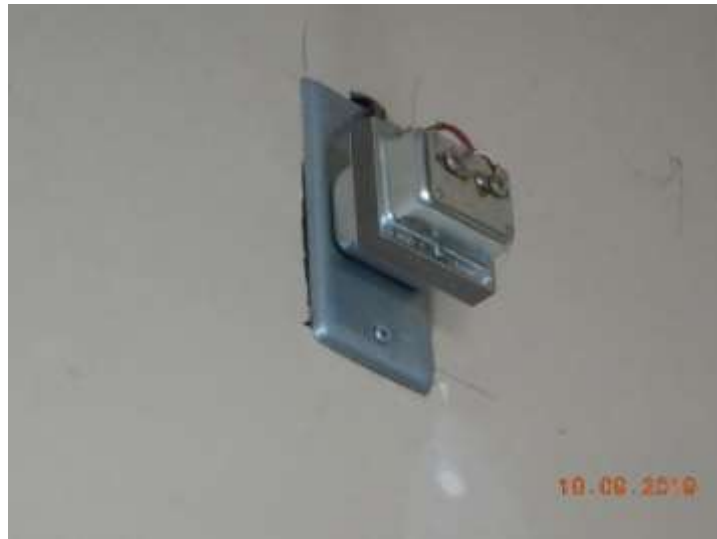
The doorbell transformer is located in the garage
