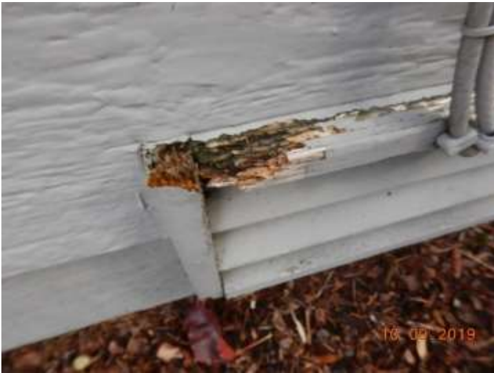
Deteriorated crawlspace vent
