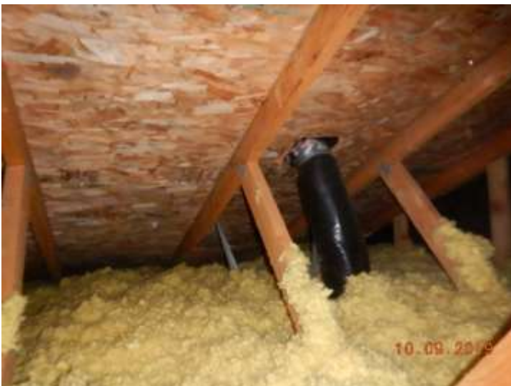
Bathroom ventilation duct
