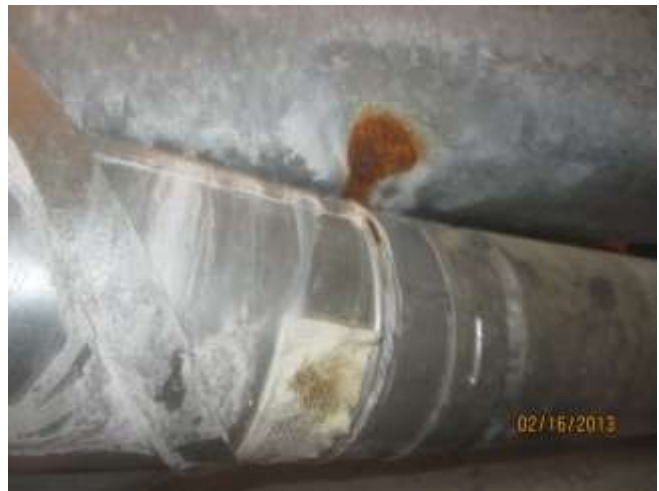
Rusting at the fresh air intake
