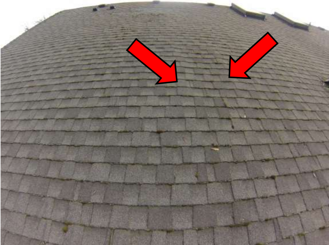
Visible sag in the roof sheathing above the Master bedroom
