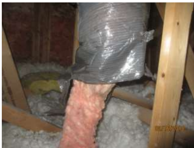
Disconnected bathroom ventilation duct
