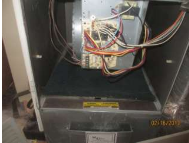
Furnace filter location
