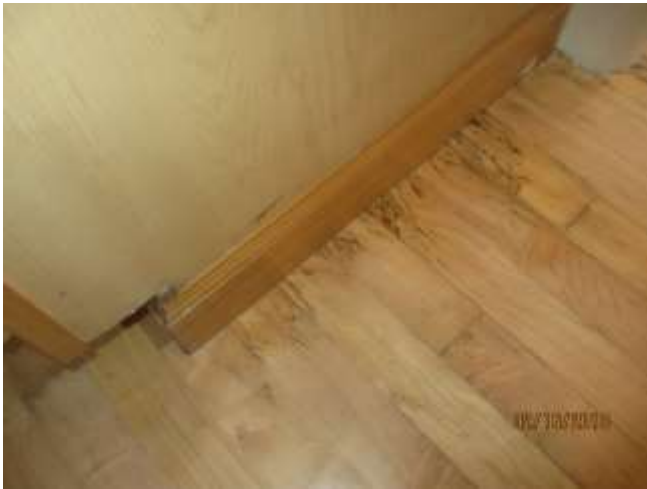
Moisture damaged hardwood floors
