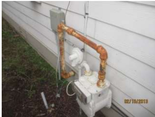
Rusting gas pipes
