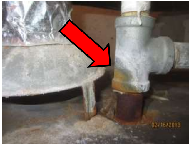
Evidence of combustion gas spillage
