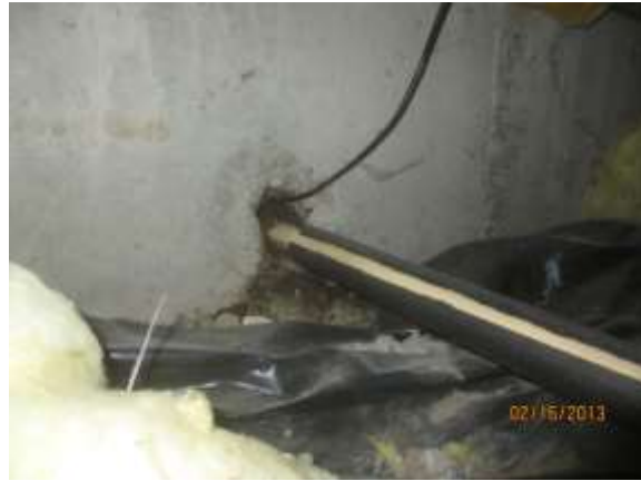
CPVC domestic water pipes
