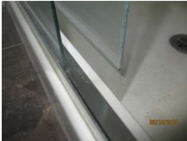
Missing shower door guides
