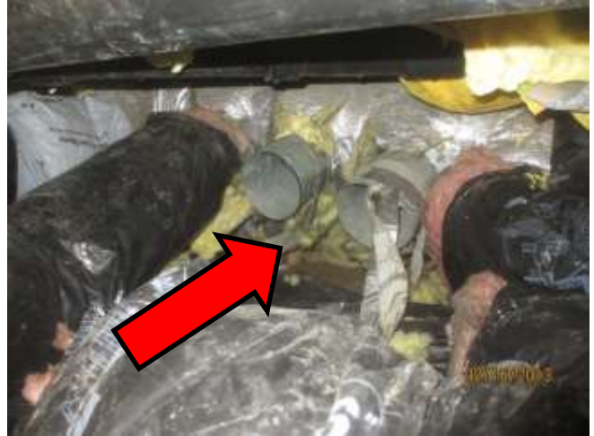
Disconnected heating ducts
