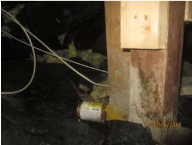
Moisture stains below the main bathroom
