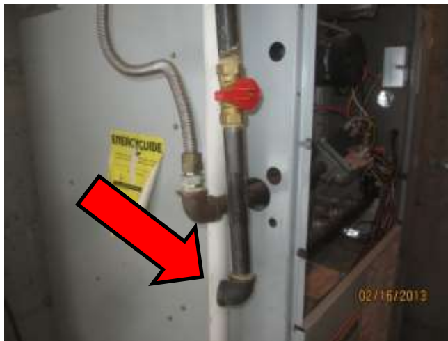
Open ended gas pipe
