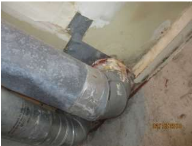
Rusting at the fresh air intake
