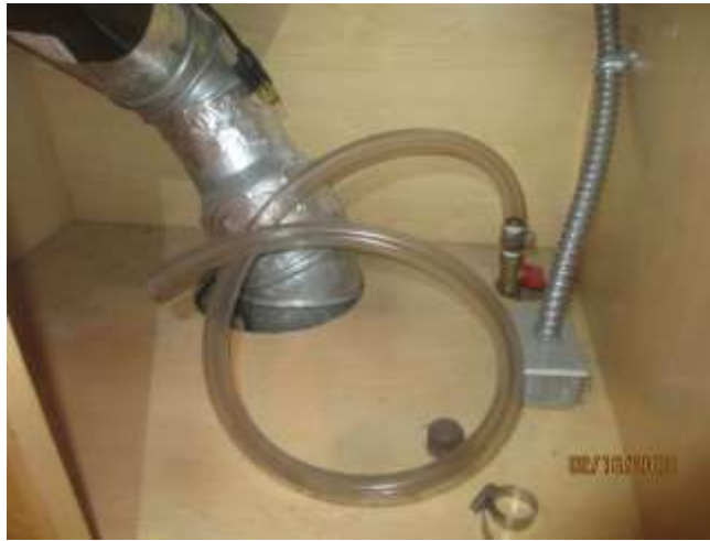
Uncapped gas line. The gas line extension is not proper
