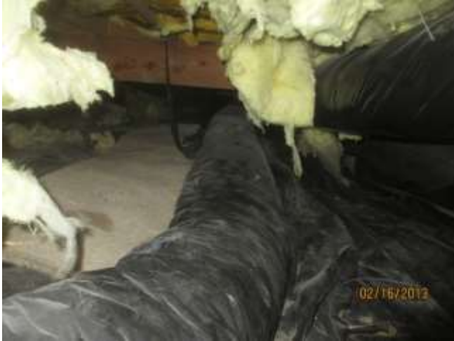
Moisture saturated heating duct
