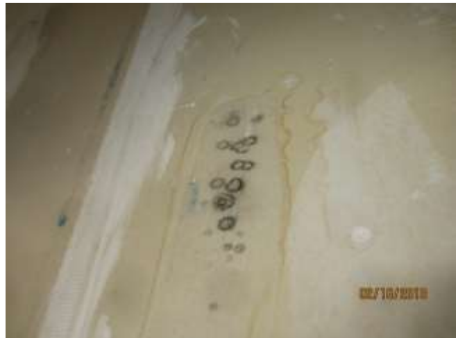
Moisture stains and mold at the South wall
