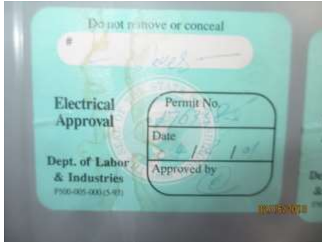
Service approval tag on the panel
