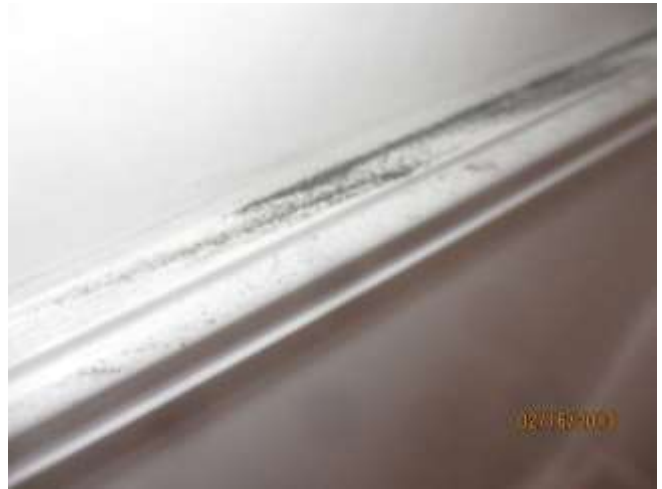
Evidence of microbial growth (mold)
