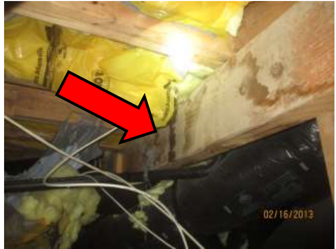
Active leakage below the floor 1 main bathroom
