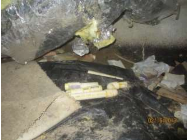
CPVC pipe repair remnants
