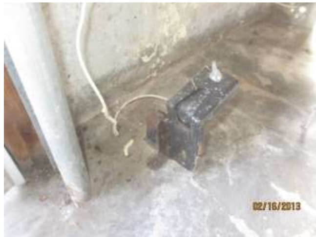
Loose photocell sensor
