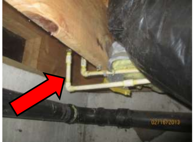
Leakage at the Kitchen sink area
