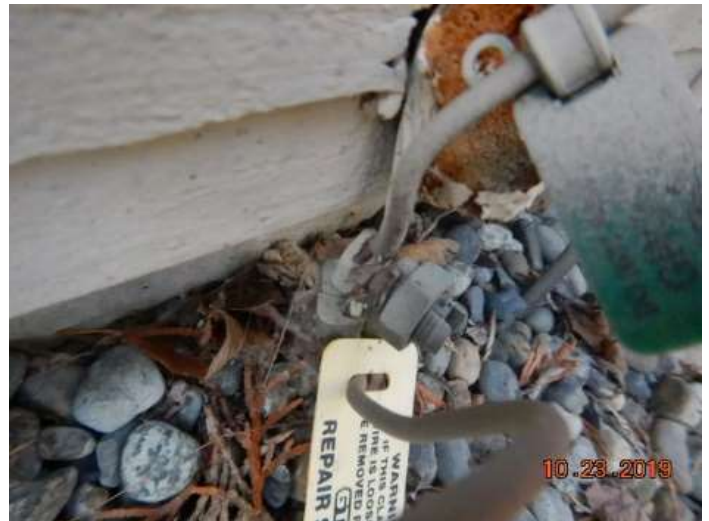
Electrical system grounding
