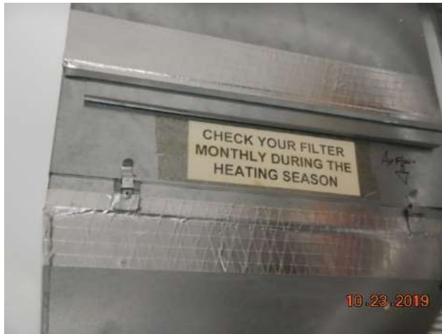
Furnace filter location
