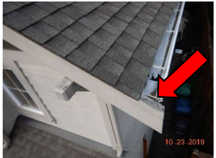
Exposed fascia board tail (typical)
