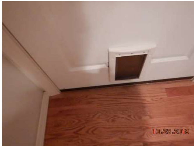
Pet door cut into the garage-house door
