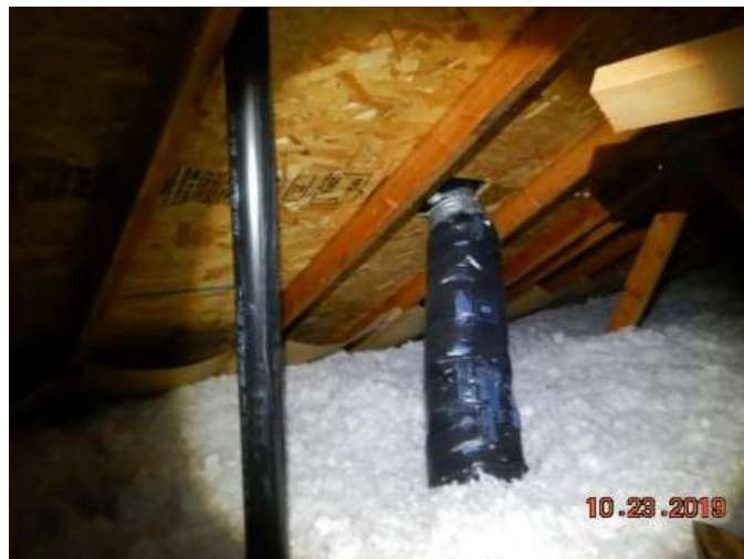
Bathroom ventilation duct
