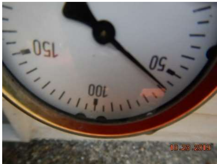
Water pressure is adequate and not excessive
