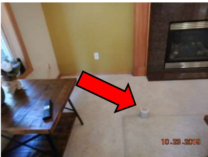
Approximate location of the leak (above) in relation to the fireplace
