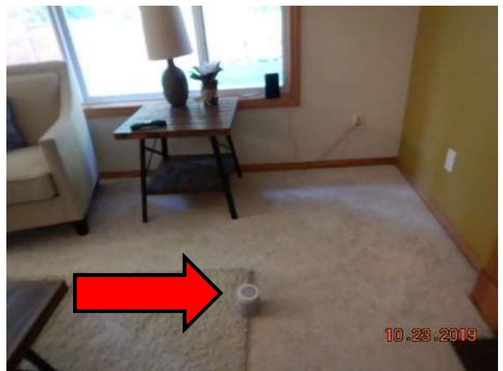
Approximate location of the leak (above) in relation to the window
