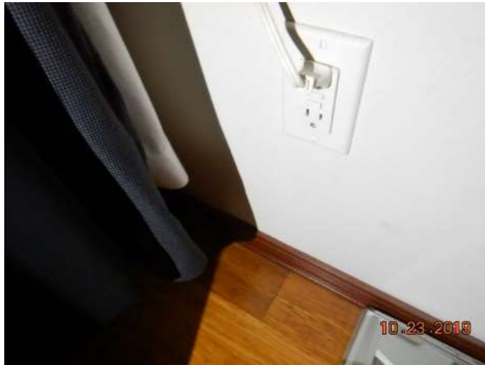
The tub motor is protected by the GFCI outlet located in the bedroom closet
