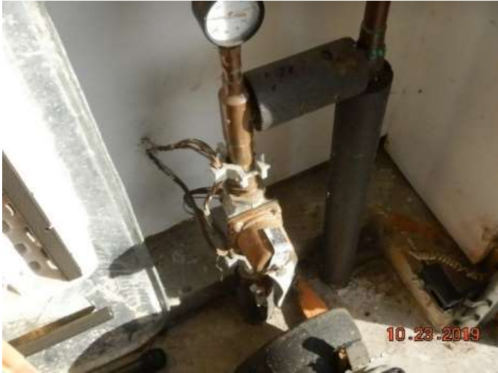
Domestic water shut off
