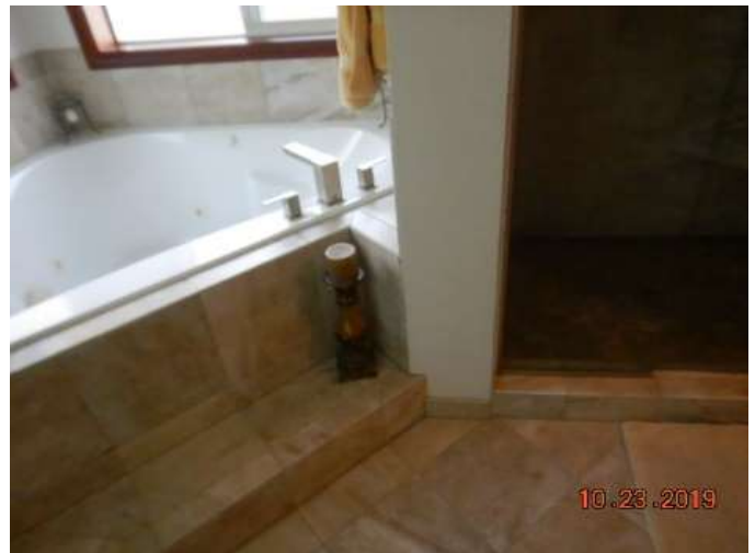
The leak appears to originate at the tub/shower valve area
