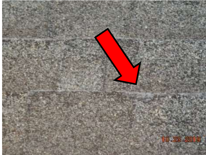
Age related wear to the lower edge of the shingles
