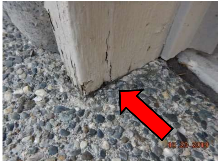
Wood rot at the garage wrap
