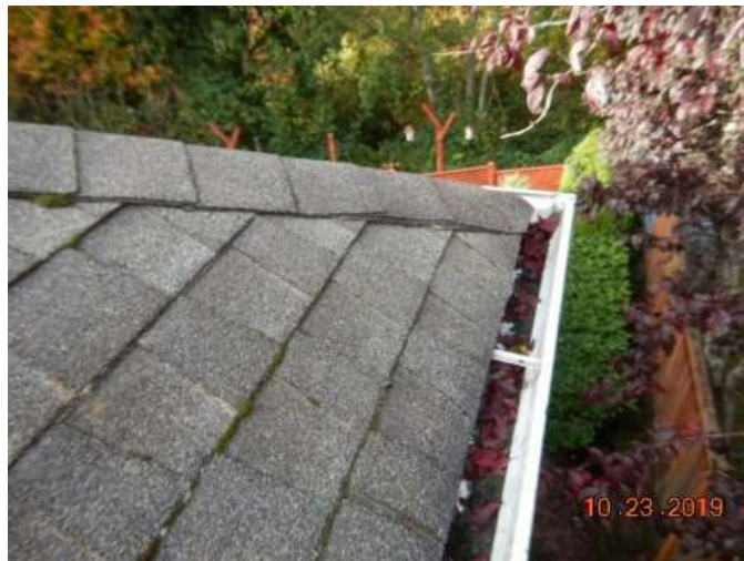
Minor debris in the gutters
