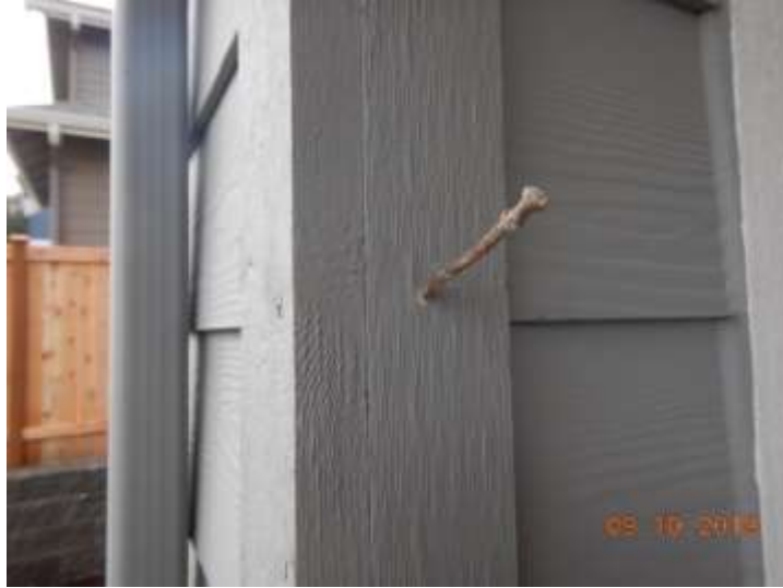
Nail protruding (typical)
