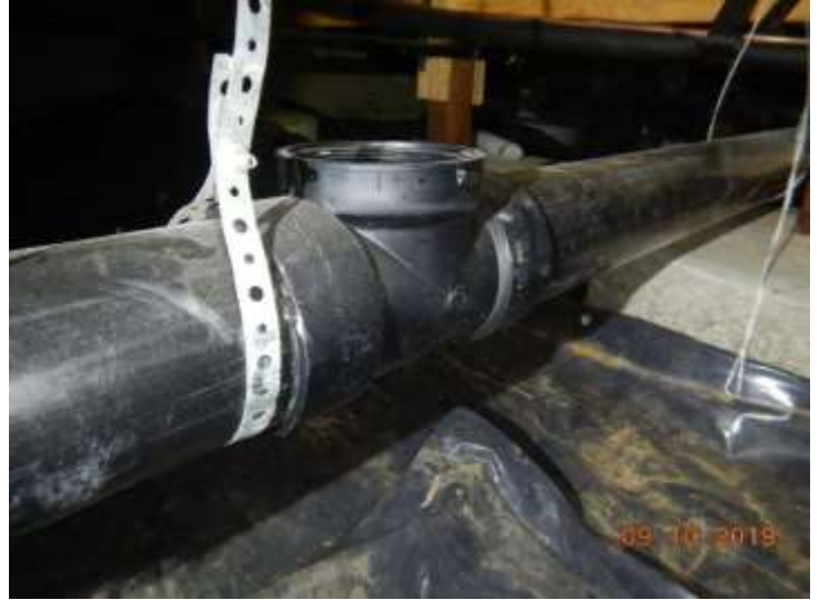
Waste line with missing cap
