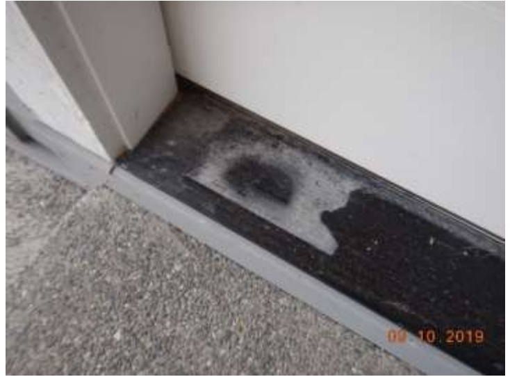
Threshold needing touch up
