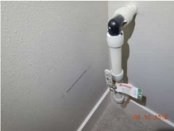
Domestic water shut off
