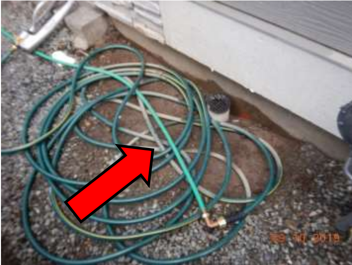
Reverse grade (ground slopes towards the house) (WDO conducive condition)
