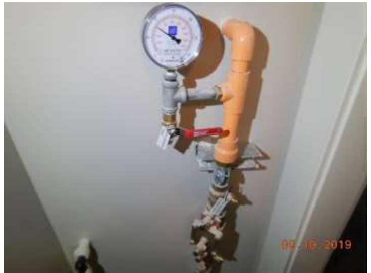
Fire suppression system
