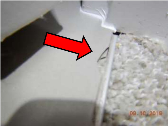
Chipped floor tile
