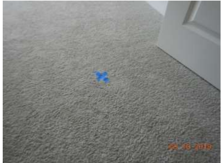
Depression at the flooring/pad
