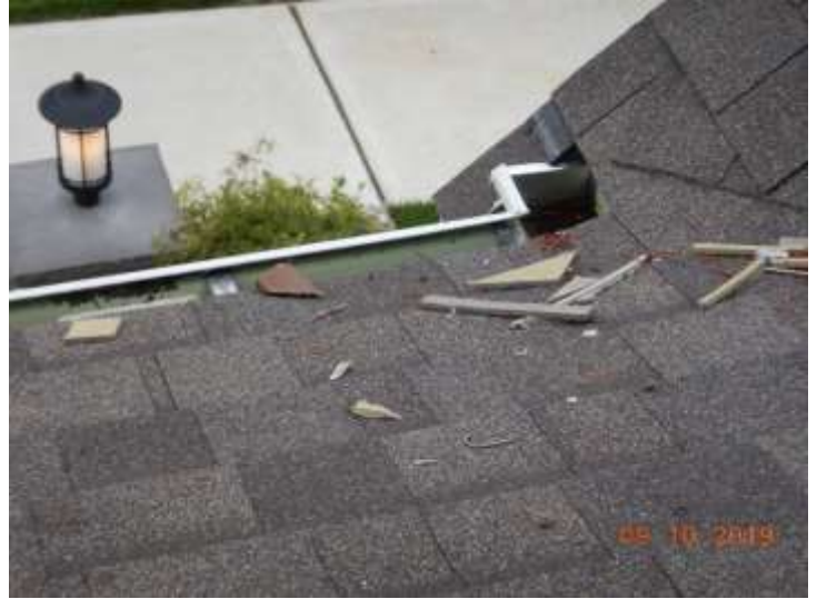
Debris on the lower roof and gutters
