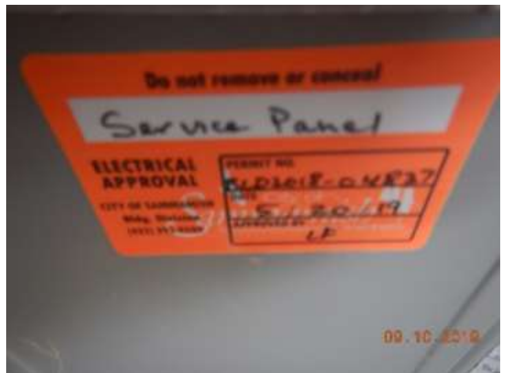
Electric service permit tag
