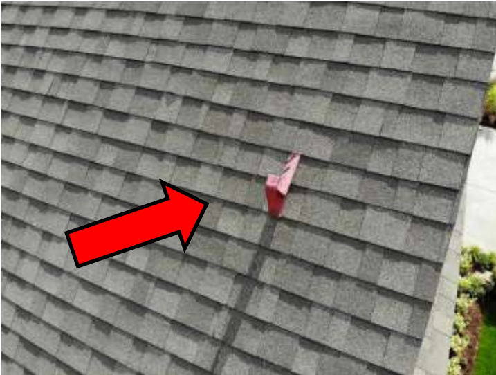
Metal anchor left on the roof
