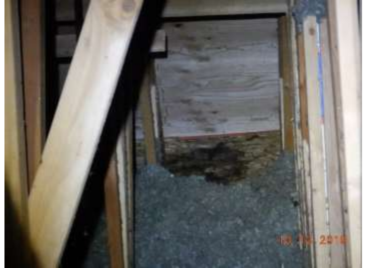
Evidence of prior roof sheathing repair at the Living room area. The roof appears to be “newer”
