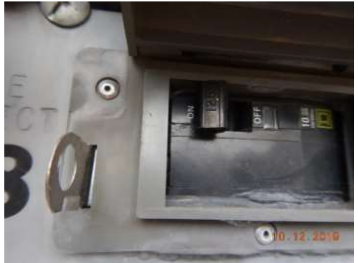
Electrical system disconnect
