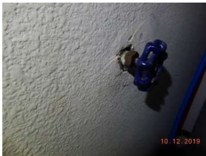
Domestic water distribution pipes
