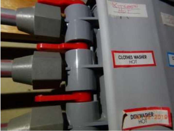
Domestic water supply pipe
