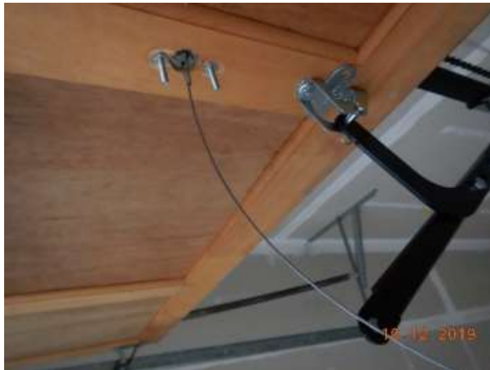
Cable attached to the emergency access key port
