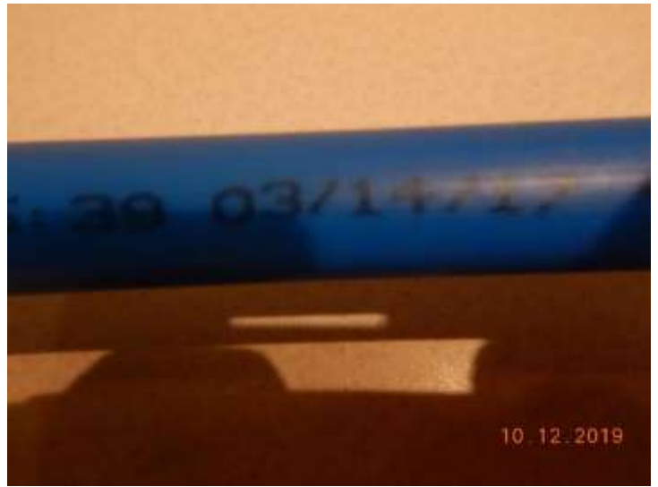
The pex pipe is dated 3/2017
