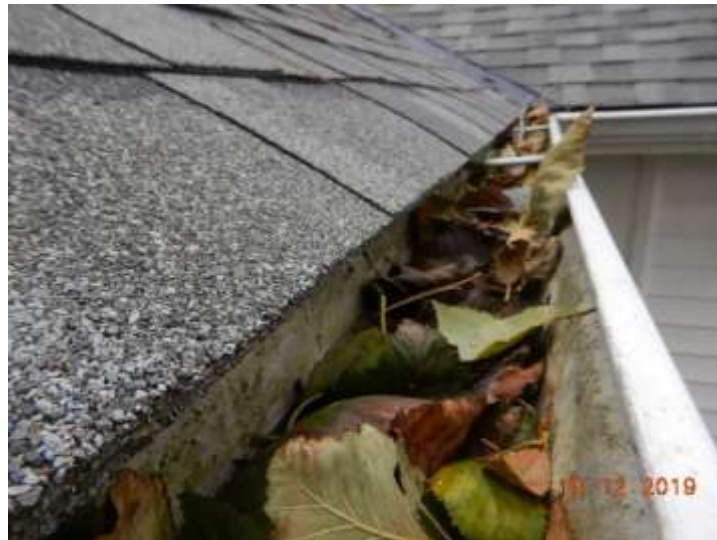
Debris in the gutters
