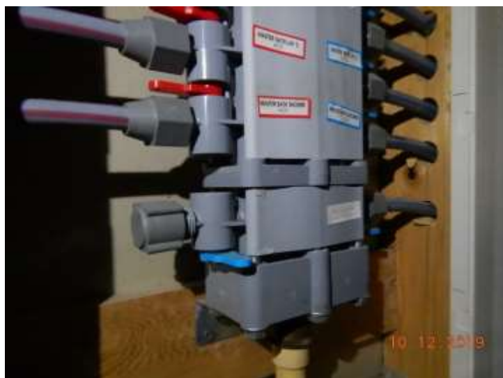
Domestic water shut off
