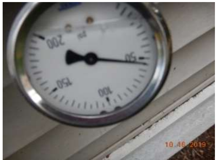
Water pressure is adequate and not excessive
