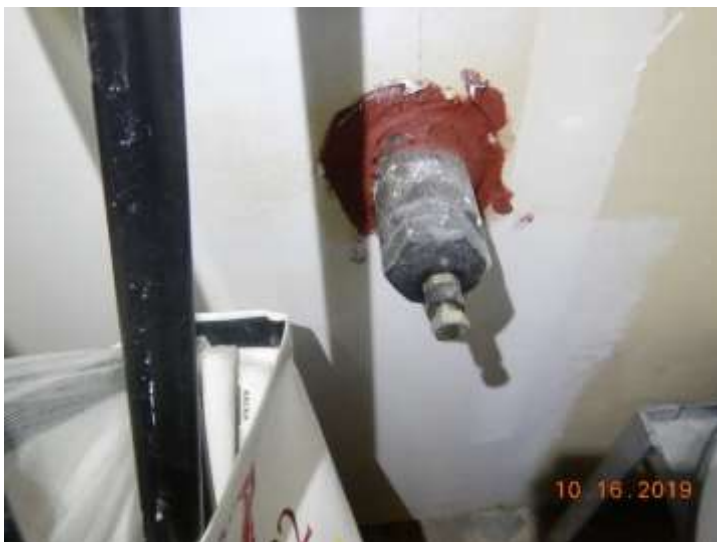
Pressure reducing valve
