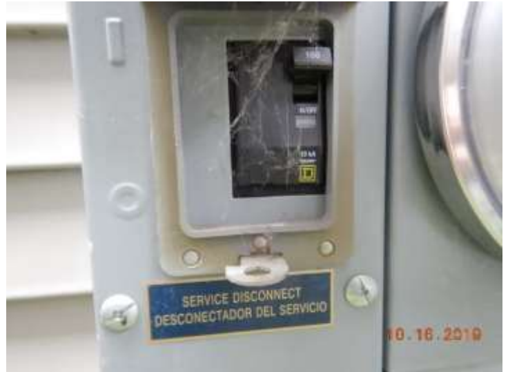
Main exterior disconnect
