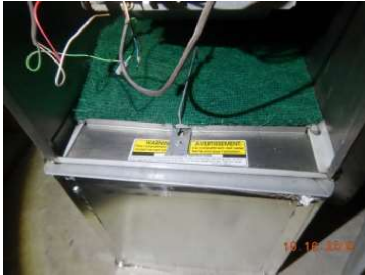
Furnace filter location
