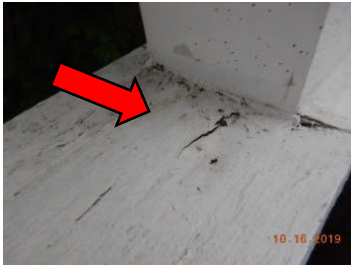
Evidence of wood rot
