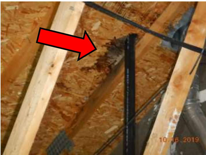
Evidence of moisture seepage
