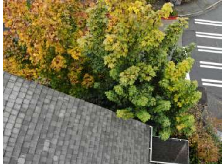
Vegetation in contact with the structure (WDO conducive condition)
