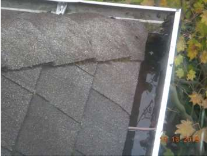
Water and debris inside a gutter
