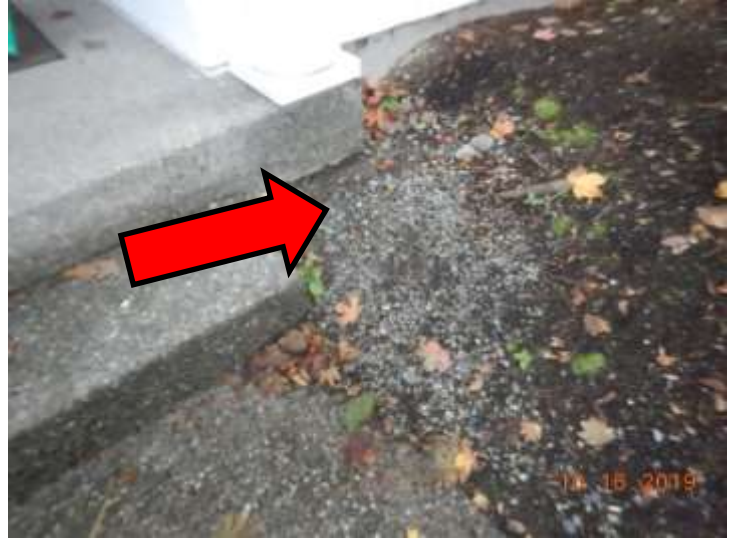
Evidence of possible gutter spillage and/or clogged drain
