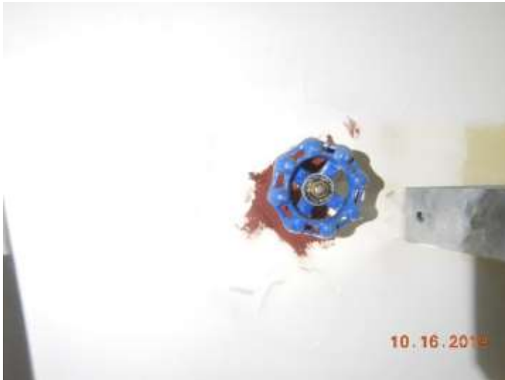
Domestic water shut off
