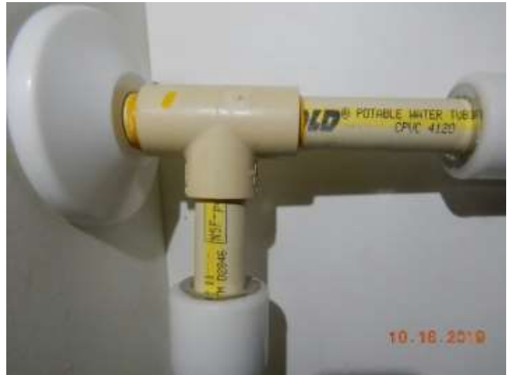
Domestic water distribution pipes
