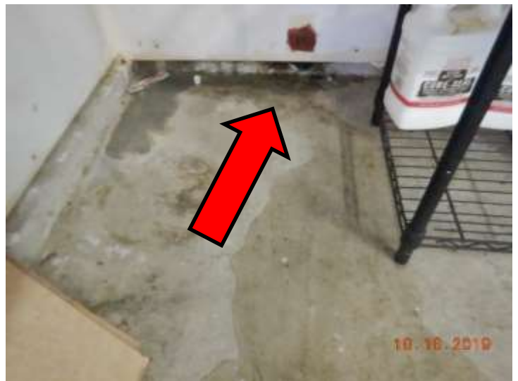
Water poured from the wall when the shut off valve was turned to the on position
