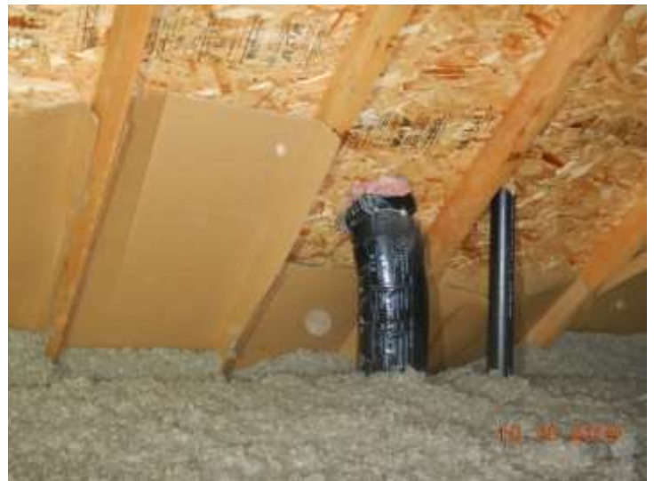
Bathroom ventilation duct
