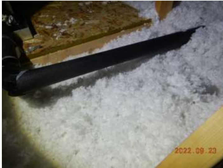
A solid platform is not installed
