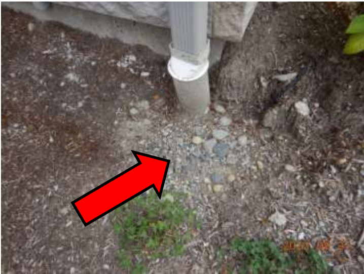
Evidence of downspout and/or drainage system spillage
