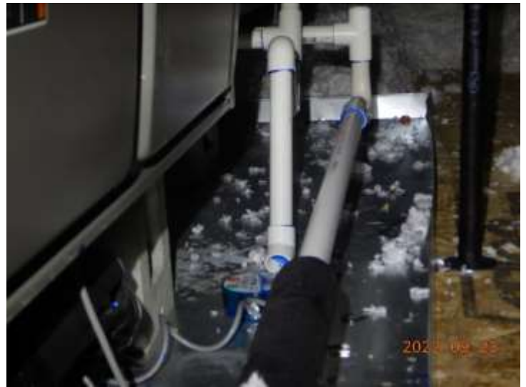
Debris in the drip pan
