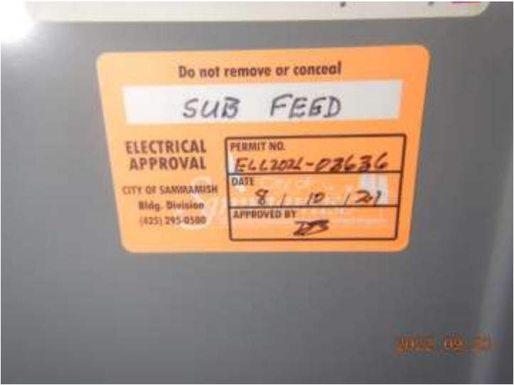
Electric service permit tag
