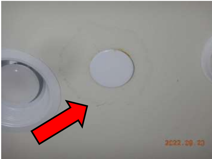
Moisture stains at the fire head
