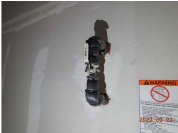
A cold weather shut off valve for the front hose bib is located in the garage
