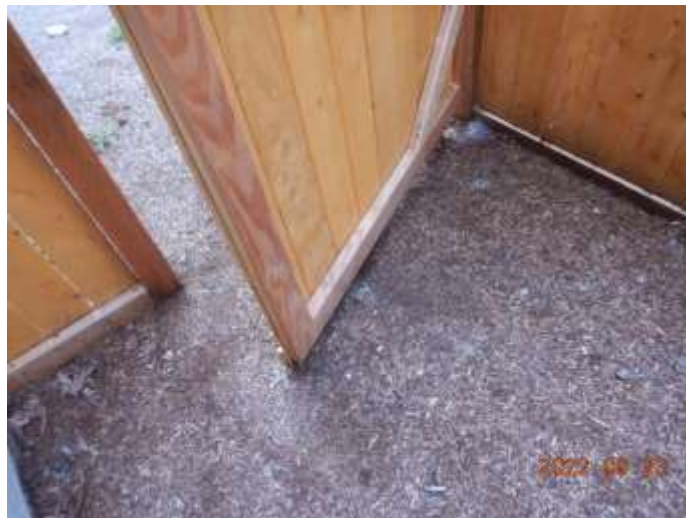
The North gate does not fully open
