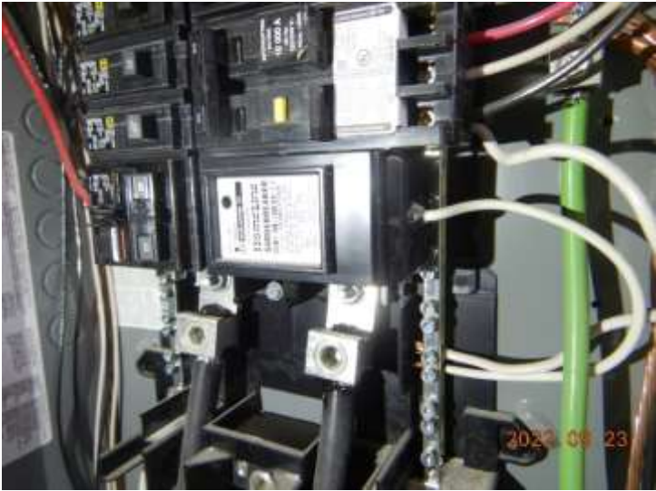
A surge protector is located at the electrical panel
