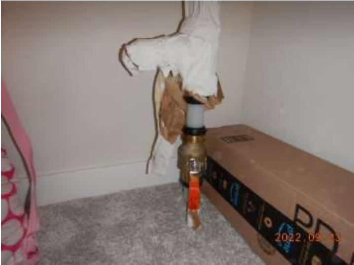
Domestic water shut off
