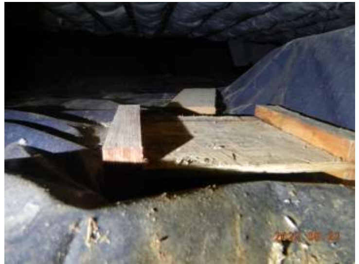
Crawlspace debris (typical)
