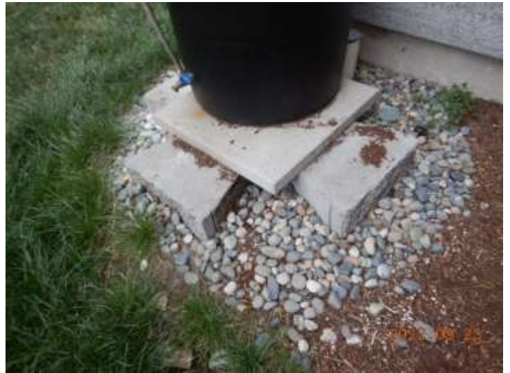
Supports for the rain barrel
