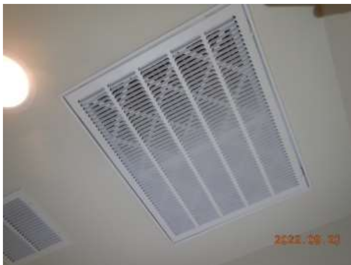
Furnace filter location
