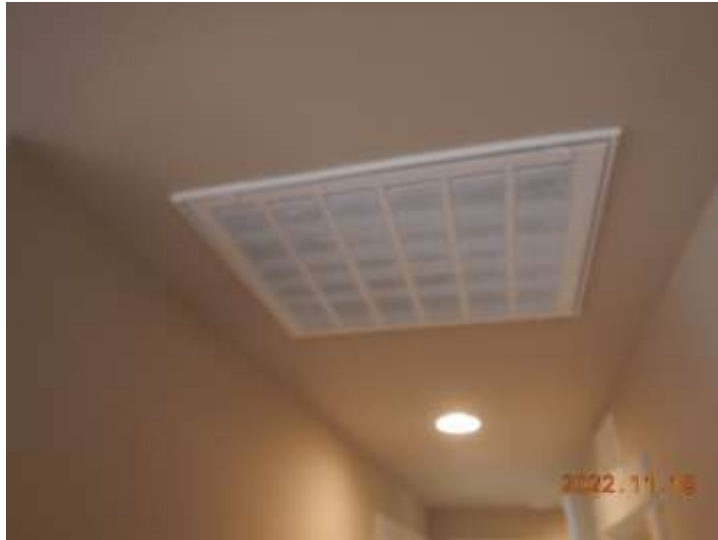
Furnace filter location
