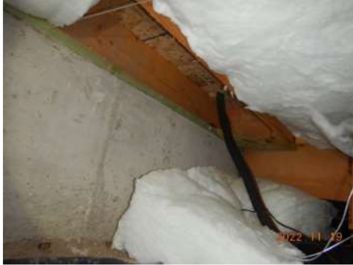
Missing underfloor insulation
