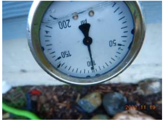
Water pressure is excessive (> 80 PSI)
