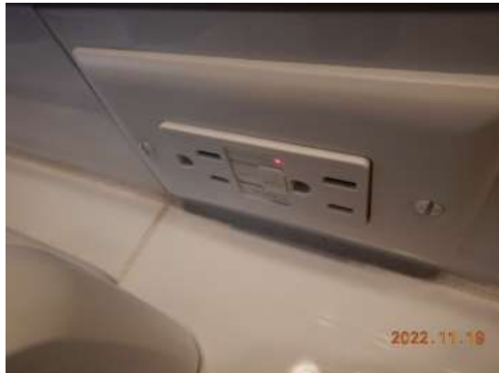
This GFCI reset outlet is the reset outlet for all of the bathroom electrical outlets throughout the home
