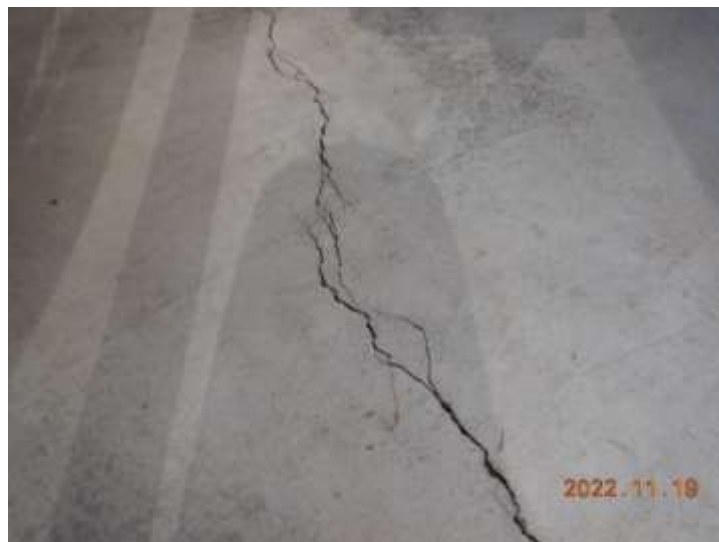
Crack at the garage slab
