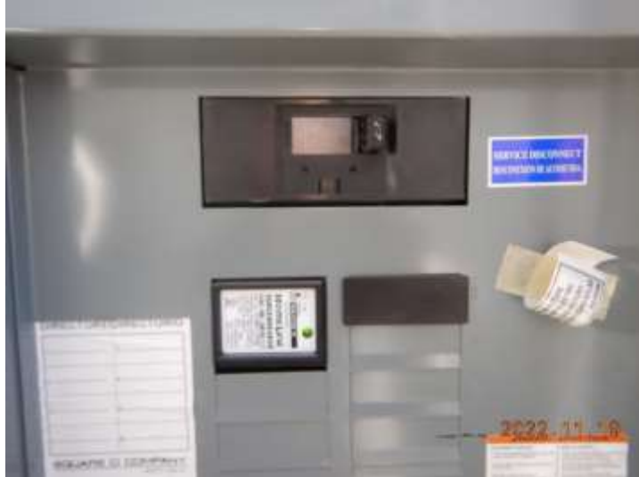
Exterior electrical disconnect
