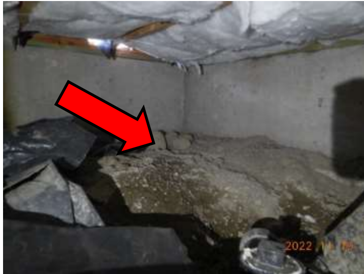
Missing vapor barrier
