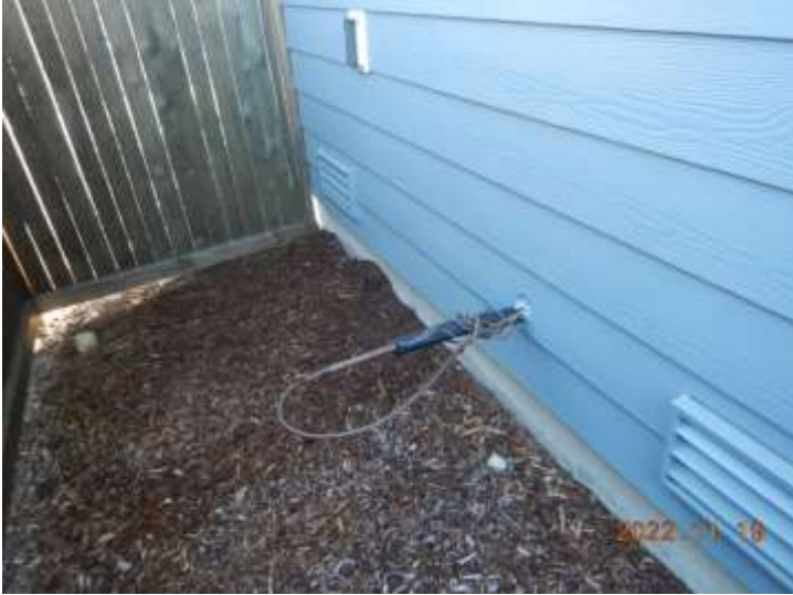
The a/c system is rough in only
