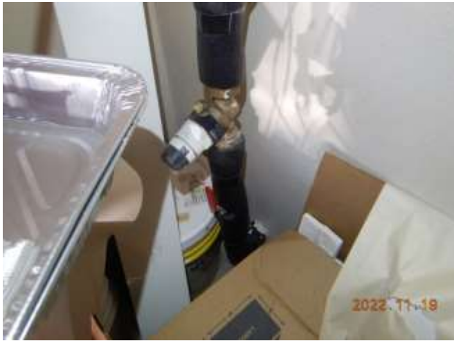
Domestic water shut off valve and pressure reducing valve
