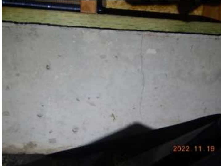
Minor crack at the foundation wall.,
