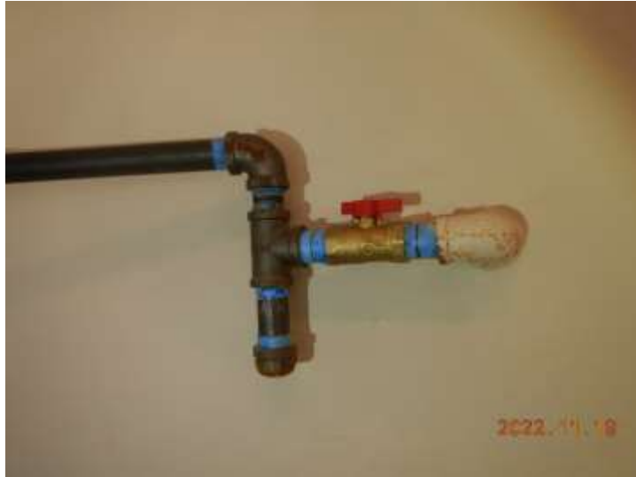
A proper gas shut off valve and sediment trap are installed
