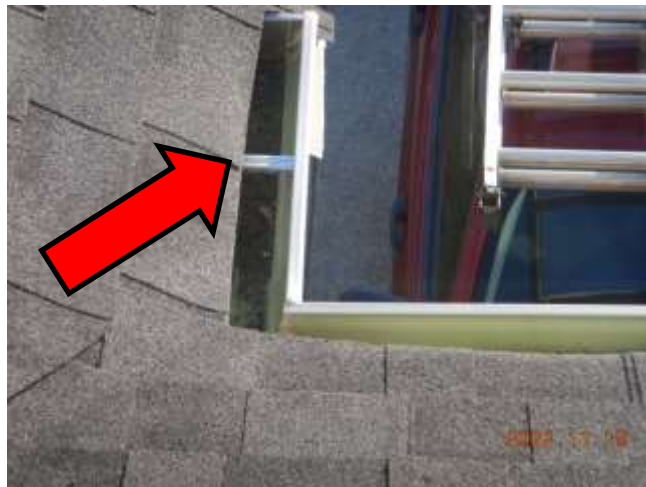
Debris build up at the gutter above the garage
