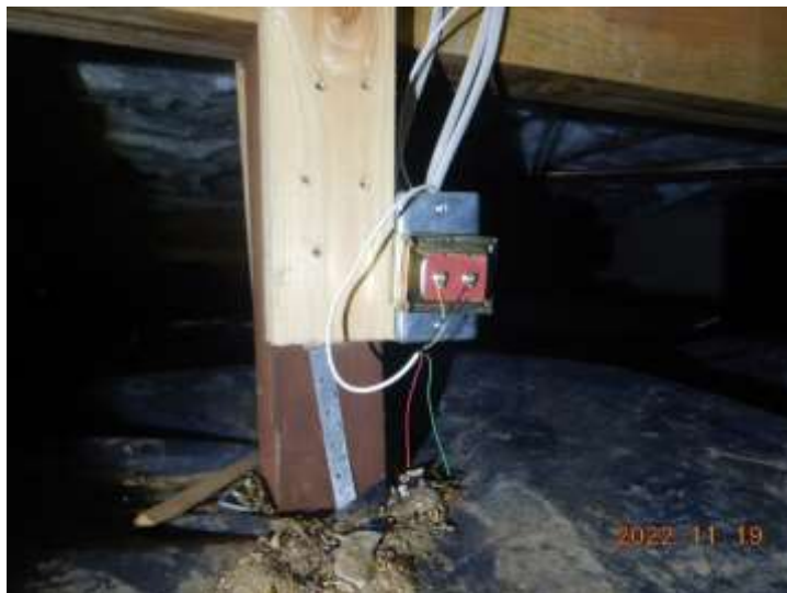
The doorbell transformer is located in the Crawlspace
