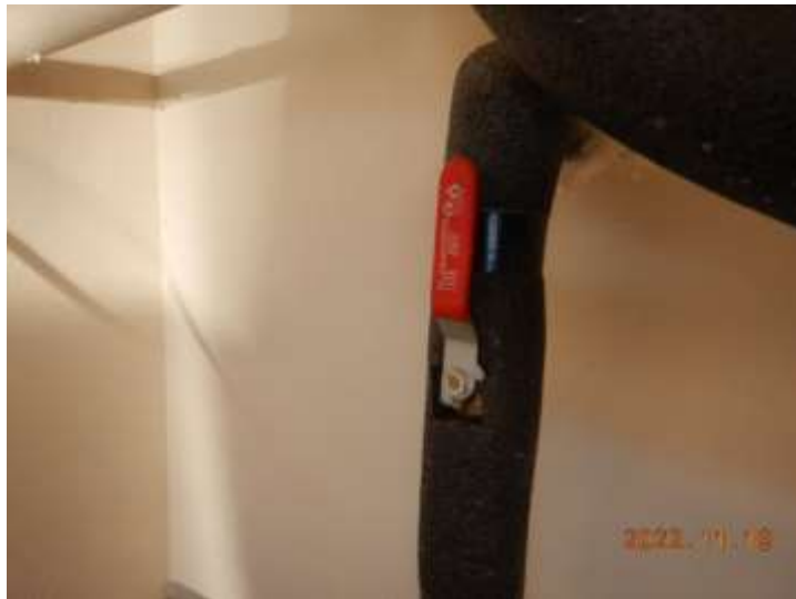
A cold weather shut off valve for the front hose bib is located in the garage
