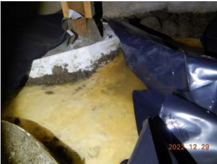
Standing water in the vicinity of the crawlspace access
