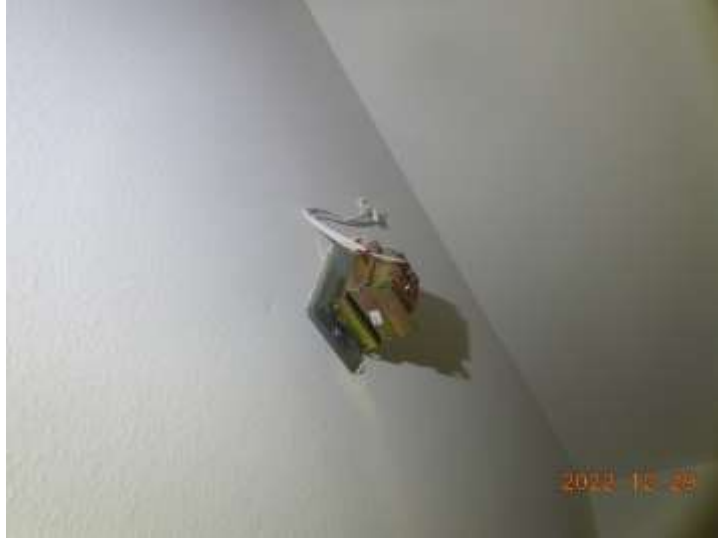
The doorbell transformer is located in the hallway closet
