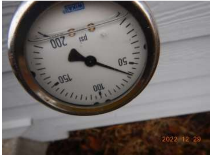
Water pressure is adequate and not excessive
