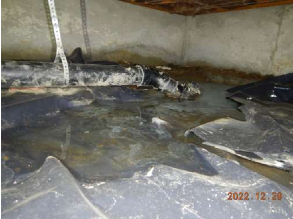
Standing water at the area below the floor 1 bedroom
