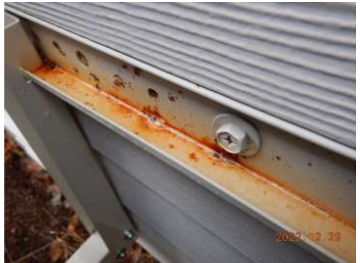
Discoloration at the exterior mounting bracket
