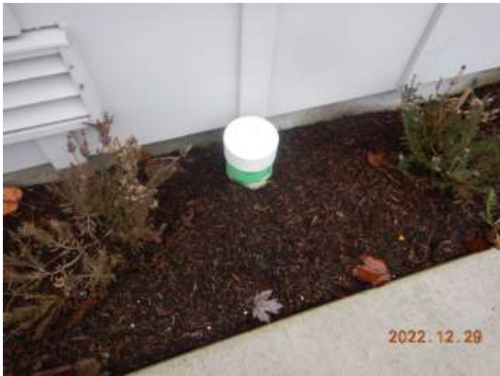
Sewer line cleanout above grade
