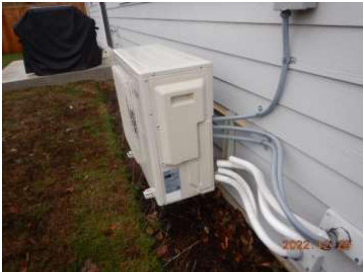
Ductless heat pump
