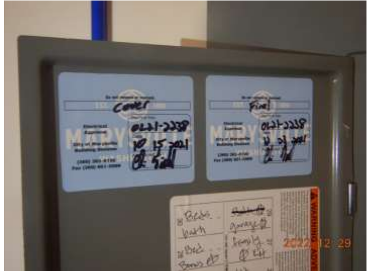
Electric service permit tag
