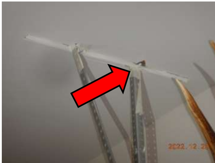
Holes at the ceiling of the garage
