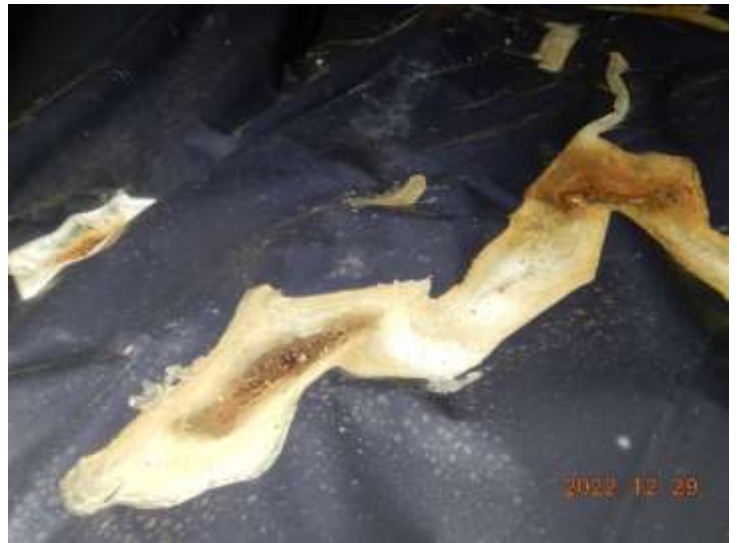
Moisture stains near a seam in the vapor barrier
