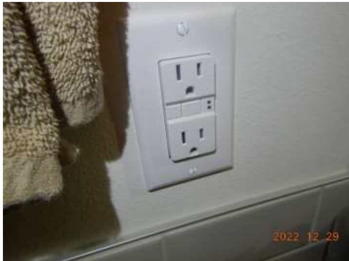
This GFCI reset outlet is the reset outlet for all of the bathroom electrical outlets throughout the home
