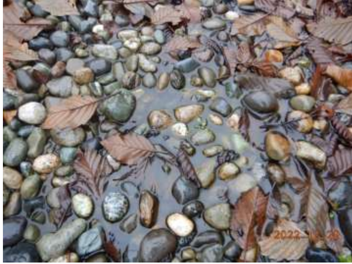
Standing water in the French drain (multiple locations)
