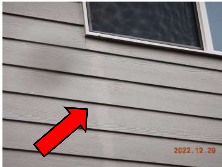
Discoloration of the paint
