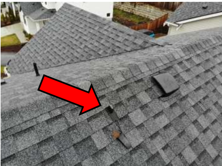
Fall protection anchor cover not installed
