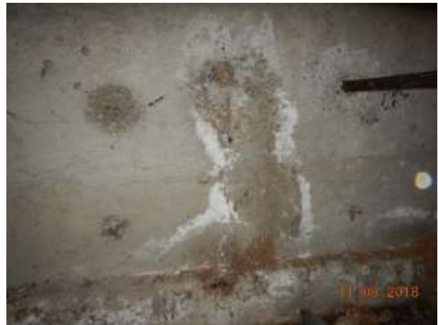
Minor area of concrete spalling off the wall
