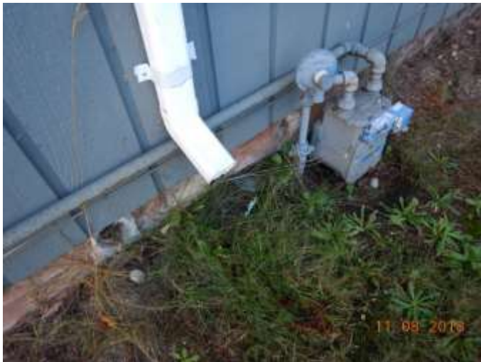
Splash blocks should be installed
