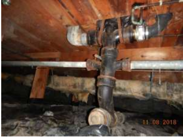
Plumbing waste lines
