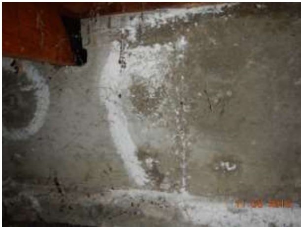
The white is evidence of excessive moisture at the exterior. No moisture intrusion is evident
