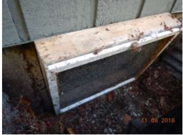
The access panel will not fit
