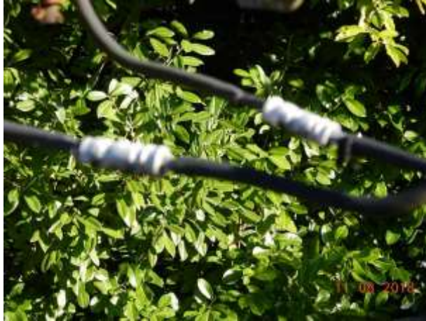
The connections are exposed
