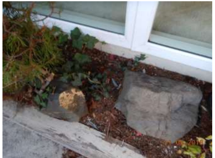
Ground in contact with the structure (WDO conducive condition)
