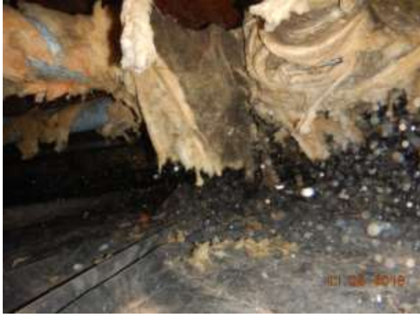
Torn insulation from rodents
