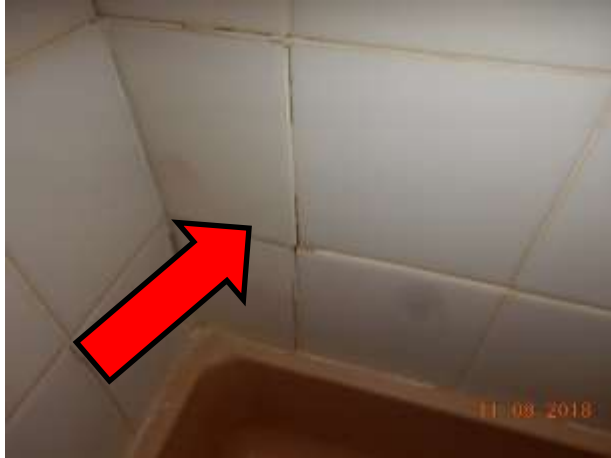
Loose tiles at the shower wall
