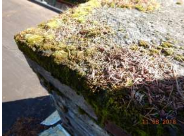
Moss on the chimney
