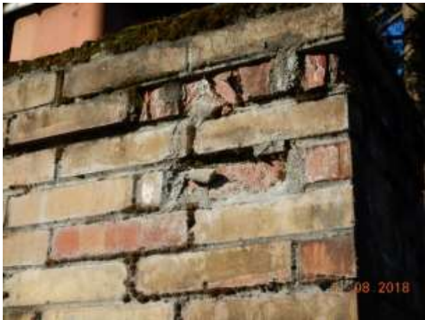
Evidence of spalling at the chimney
