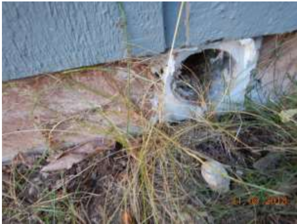
A vent flap is not installed
