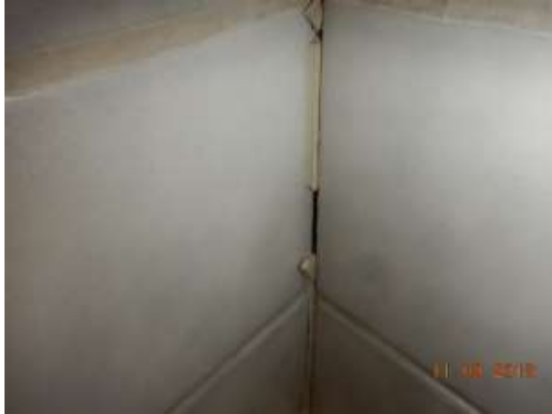
Gaps at the shower wall grout
