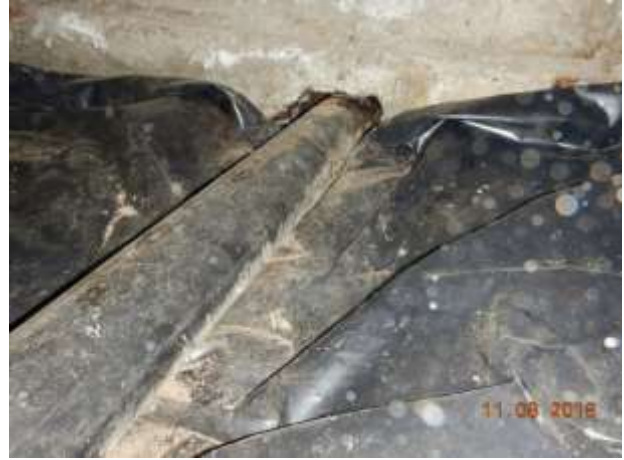
The side sewer may be “newer” as the pipe that exists the home is ABS (a newer material)
