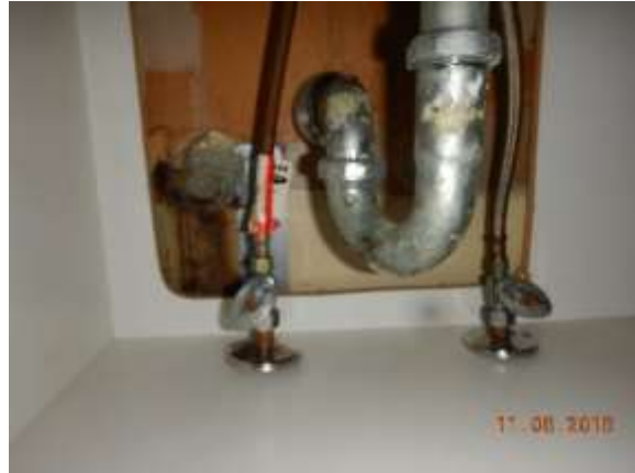
Copper domestic water pipes
