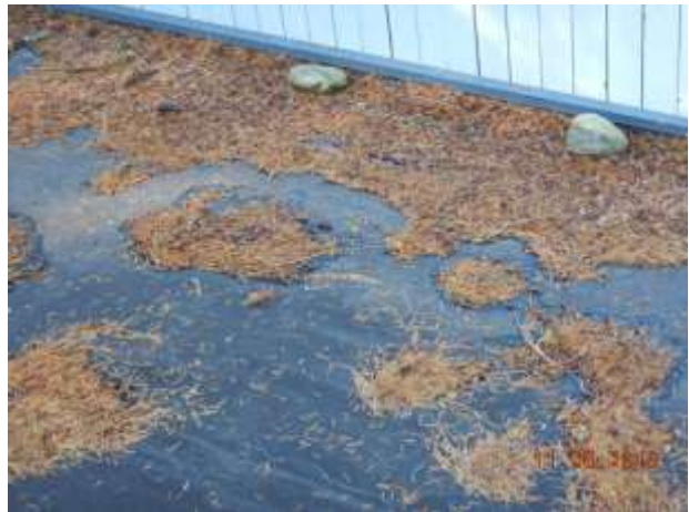
Debris on the roof
