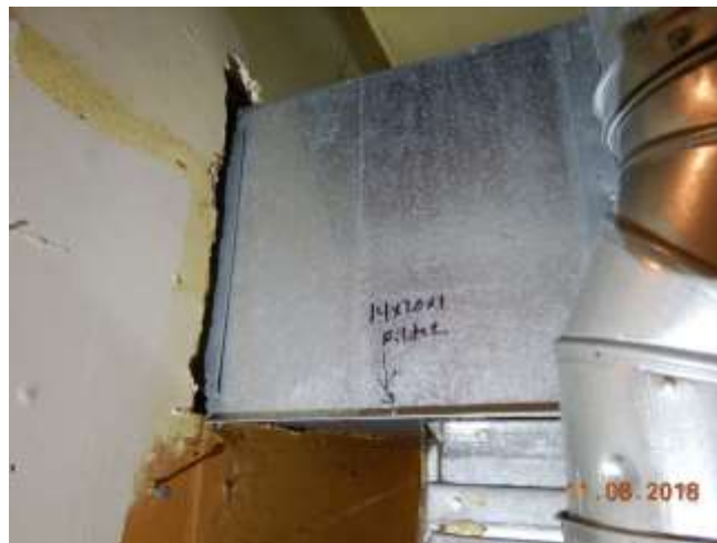
Furnace filter location
