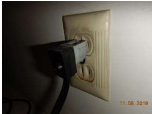
The electrical outlet for the clothes washer is not grounded
