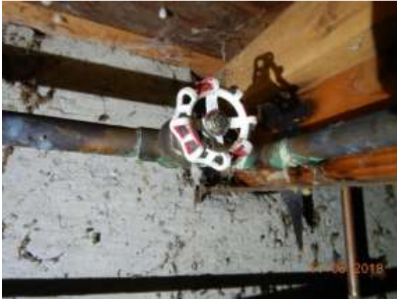
Domestic Water Shut off
