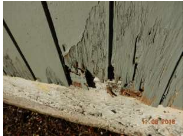
Wood rot at the garage siding
