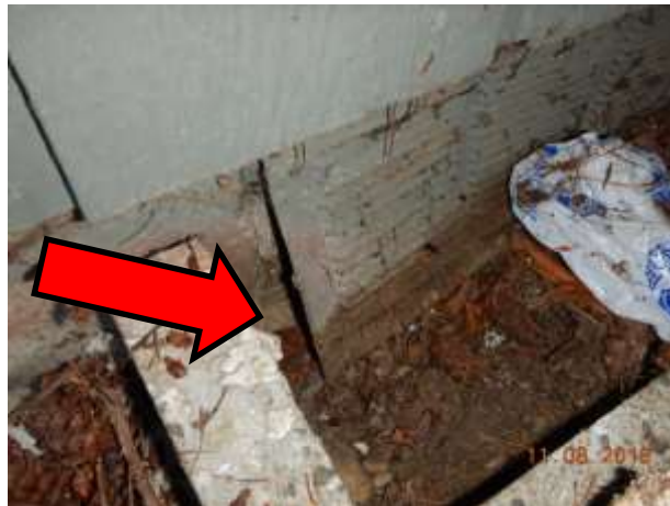
Gap at a crawlspace vent
