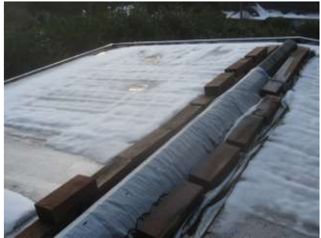
Blocked ridge ventilation
