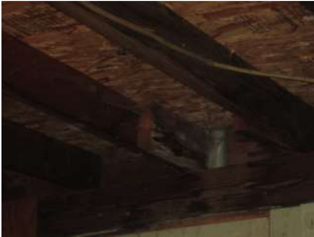
Moisture stains at area adjacent to shed
