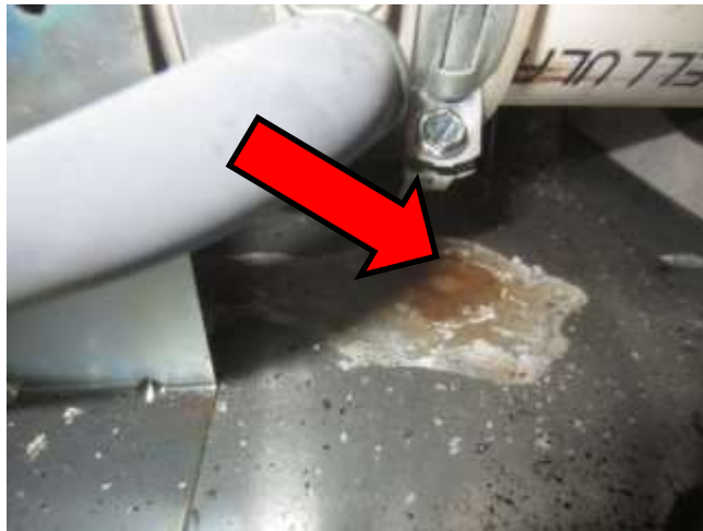
Condensate inside of furnace
