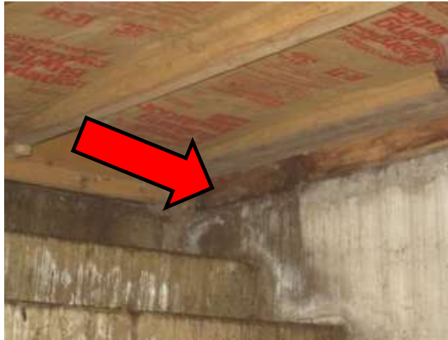
Wood rot and moisture intrusion visible
