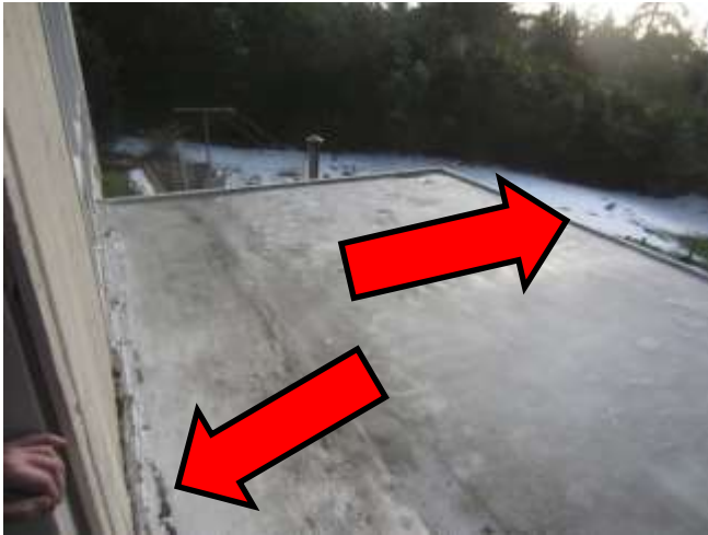
No barricade to roof above storage shed
