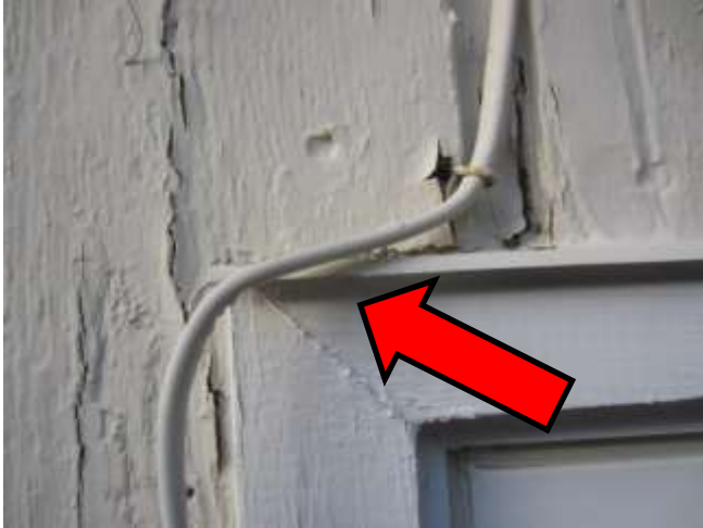
Extension cord wiring to exterior outlet
