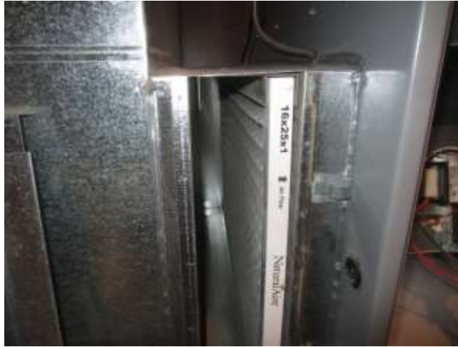
Furnace filter compartment
