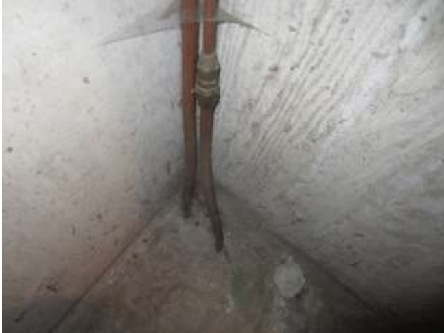
Oil tank lines in basement
