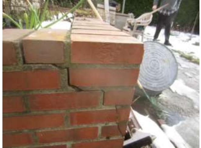
Cracks rear planter
