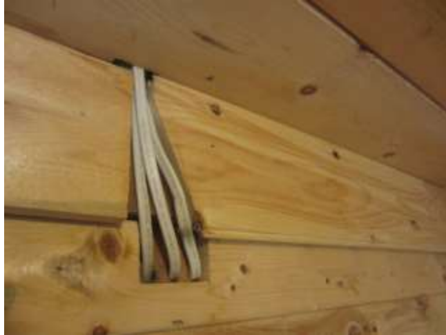
Surface mounted electrical wires
