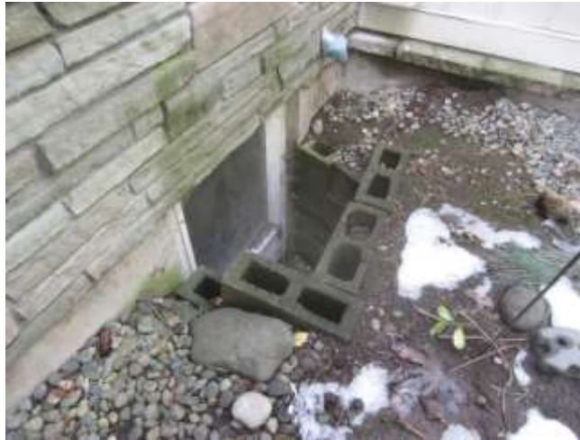
Fall hazard into window well and adjacent non-tempered glass window
