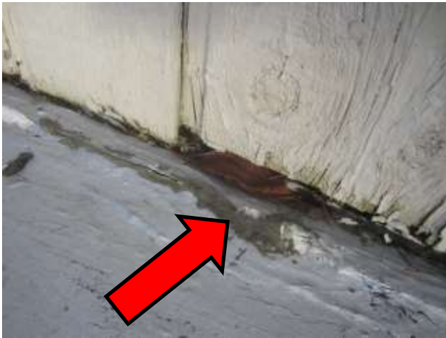
Siding to roof separation is negligible at shed roof
