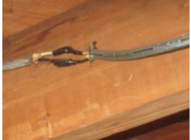
Wire splice in great room
