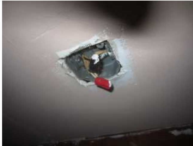
Exposed electrical wires in closet
