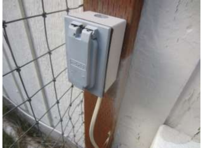
Extension cord wiring to exterior outlet
