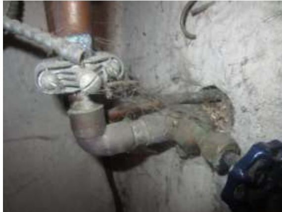
Domestic Water Shut off
