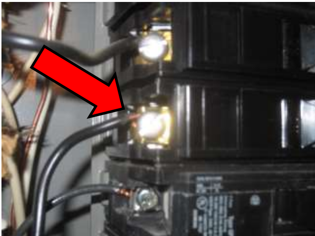
Double tapped breaker
