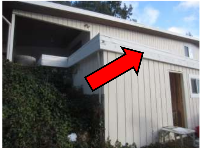
Fall hazard from storage shed
