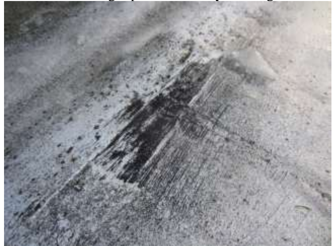
Coating is worn at roof (typical)
